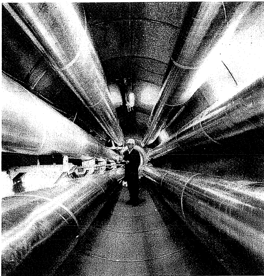
FIGURE 18.7 View into the tunnel. (Courtesy of Siemens.)
