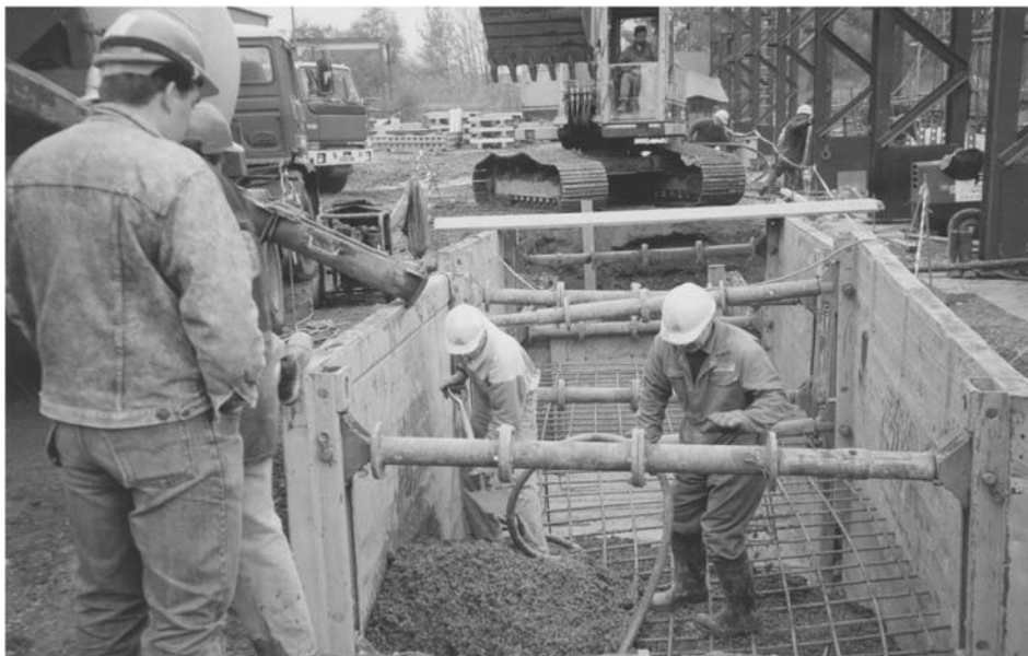
Plate 12a. On any job not properly supervised the strangest things can happen. It looks as if someone forgot the reinforcement until after the first placement of concrete. A resident engineer would stop the work and require it to be redone properly
