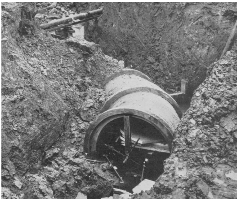
Plate 8a. Presumably somebody thought this trench was stable – and was proved wrong
