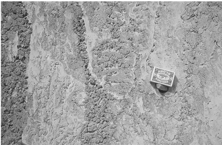
Plate 15b. Sand runs on a concrete wall surface
