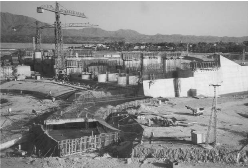
Plate 1b. Power channel inlet structure, Ghazi Barotha Hydropower project, Pakistan 1999
