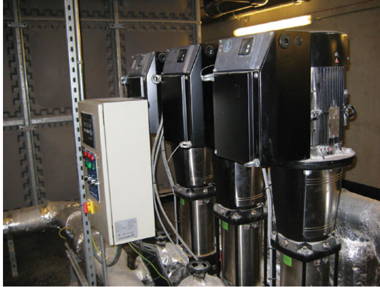
Figure 9.1 Variable speed drives
