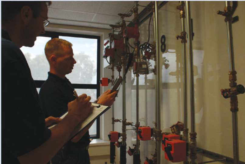
Figure 11.2 Commissioning training – example, water balancing and flow rate measurement
