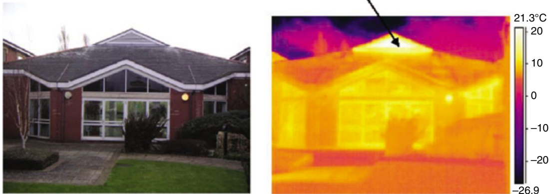
Figure T12.3 Excessive heat escaping from a building
