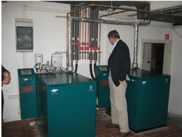
Figure 9.3 Combined heat and power
