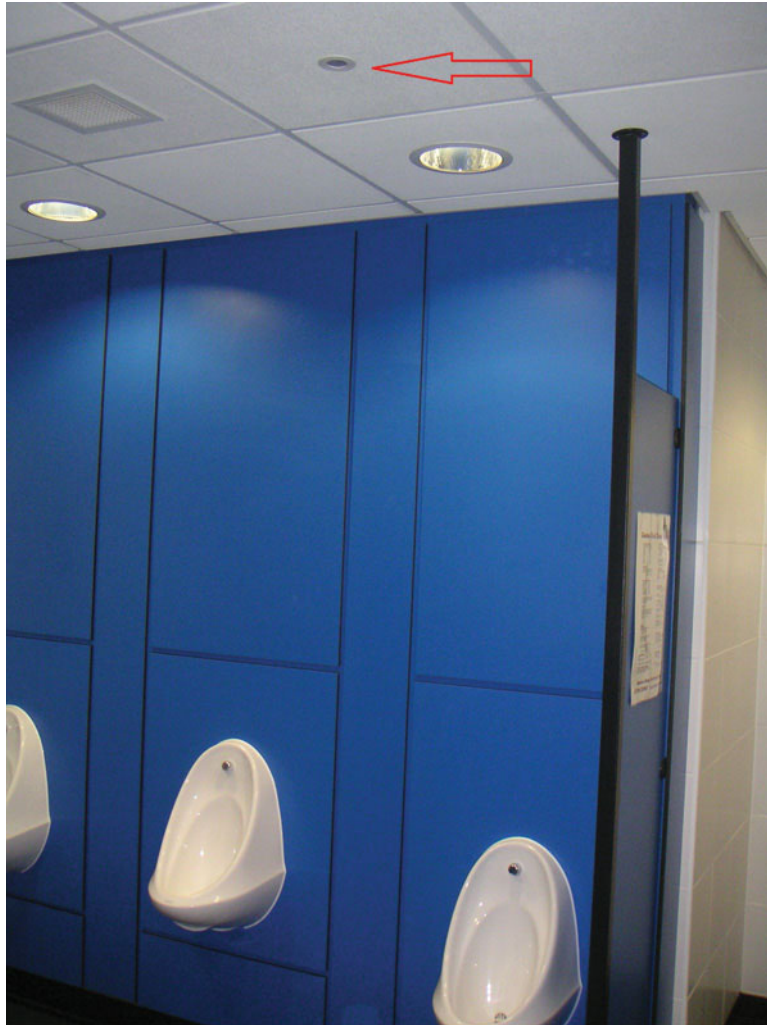
Figure 7.9 Several urinals controlled by a presence detector (as indicated) linked to an automated valve
