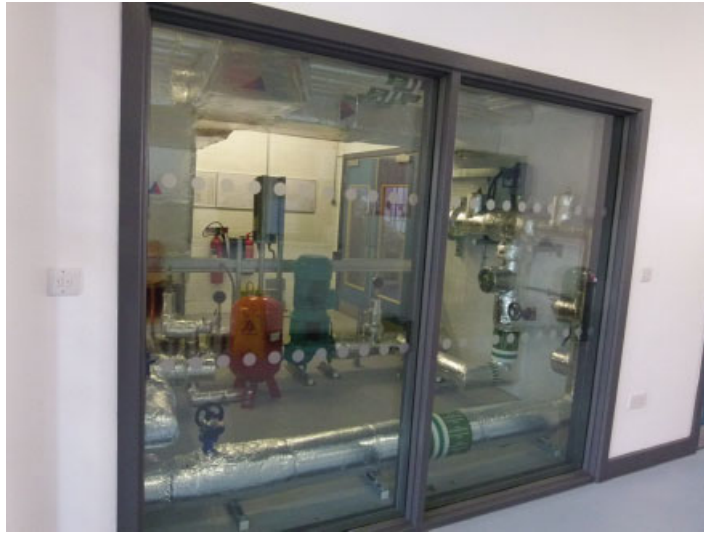
Figure 12.1 A ground-floor plant room with a viewing panel for all to see
