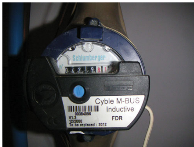
Figure 7.3 An inline water meter: can be used on the main supply in other areas in the building
