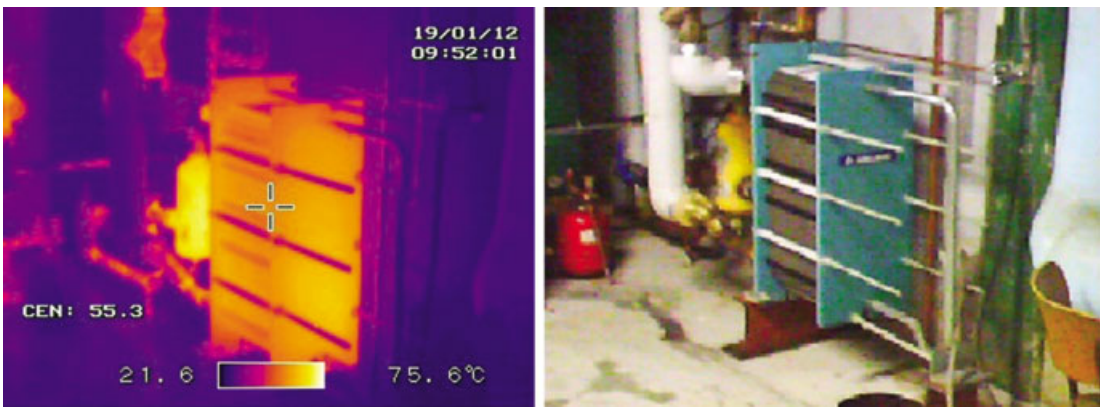
Figure T12.19 Heat exchanger uninsulated
