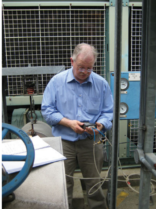
Figure 11.9 Testing and validating water flow on large chillers
