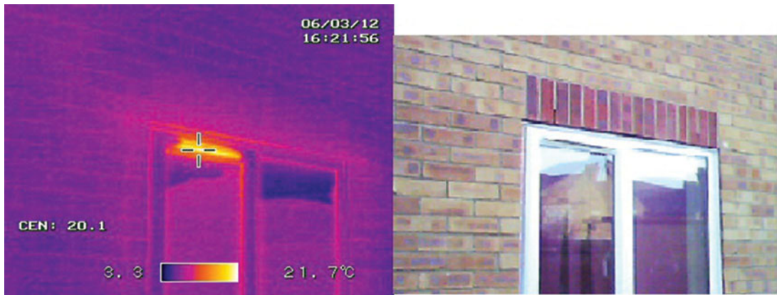
Figure 9.7 Thermal image showing heat escape via a trickle vent
