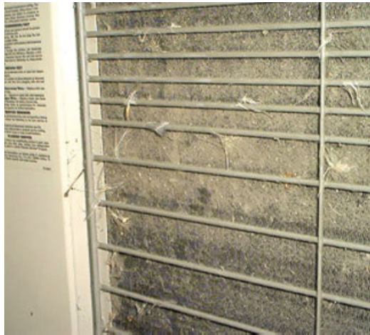
Figure 12.2 Blocked filter – bad for operation and energy performance
