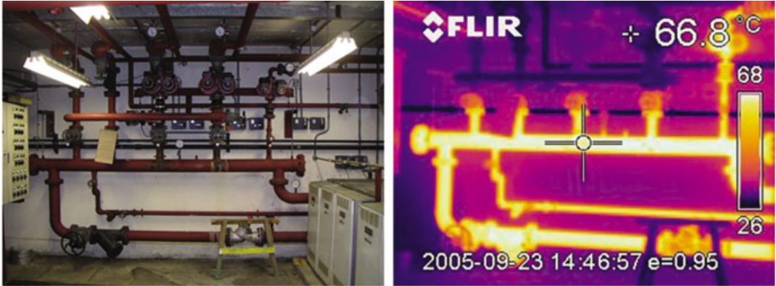
Figure T12.15 Pipework checking – insulation needed!
