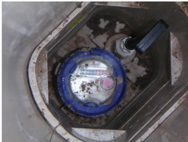
Figure 7.1 A water meter; often out of sight, out of mind
