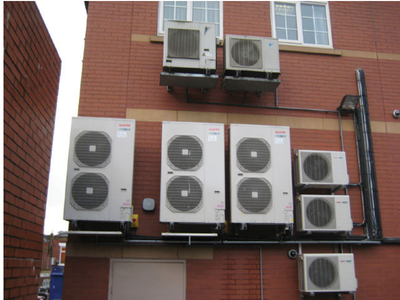
Figure 9.12 A wall of split condenser units
