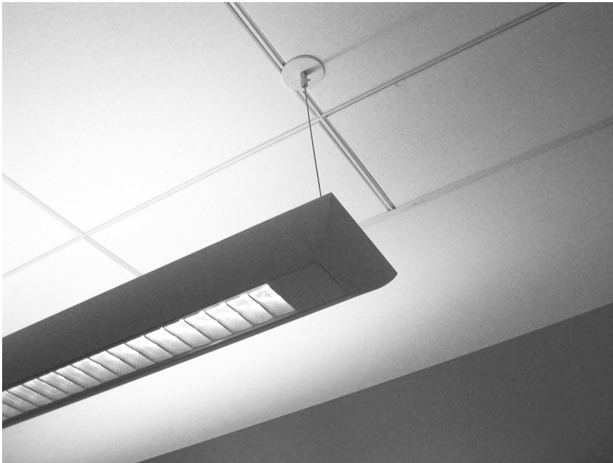
Figure 8-3. A direct/indirect pendant fixture. These often come with specifications that indicate what percentage of the lamp is projected as indirect uplight, and what percentage is direct downlight. Some come with different diffuser and reflector options that enable the user to precisely select how much of the light is indirect and how much is direct.
