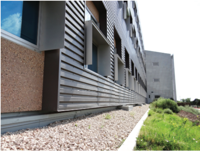
Figure 7-22. Transpired solar collector is affixed to south wall of RSF to preheat ventilation air. Visible at the bottom of the wall are the ducts that draw the preheated ventilation air into thermal storage within the concrete foundation of the building. (Photo by the author)
