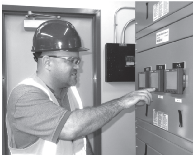
Figure 1-8. Brett Jackson at the Windsor Readiness Center, site of one of the solar energy projects that he is managing for the Colorado Army National Guard. (Photo by Michael Jaurrieta, courtesy of Colorado Army National Guard.)
