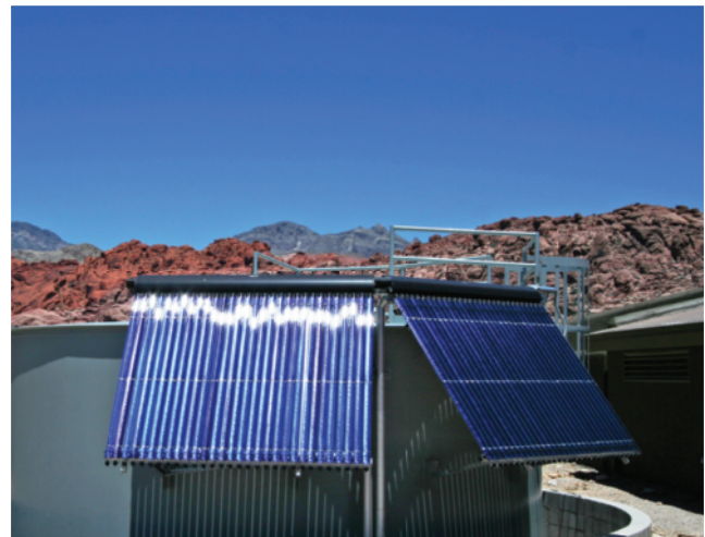
Figure 7-15. Two solar water heating evacuated tube solar collectors are mounted on a 15,000-gallon tank for harvested rainwater storage. (Photo by Henry Tom, AIA, NCARB, courtesy Line and Space LLC)
