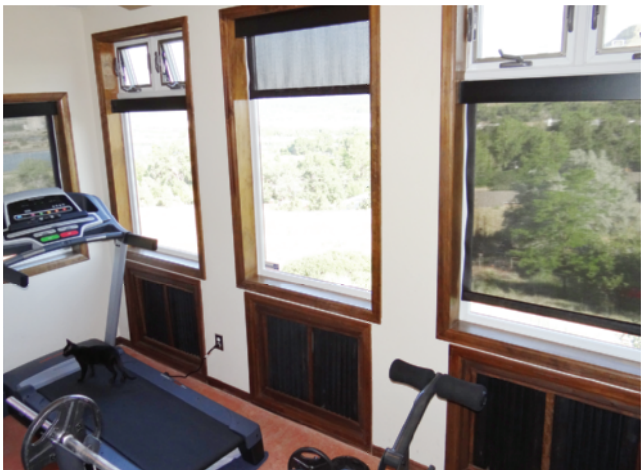
Figure 7-9. Phase change panels in thermal storage wall at solar home in Golden, Colorado. (Photo by the author)
