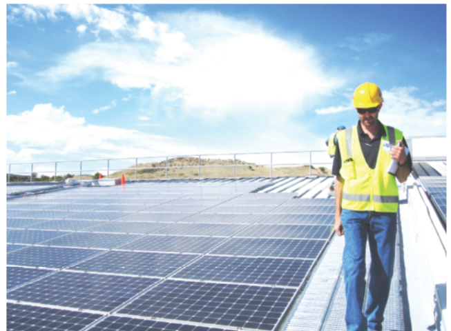
Figure 7-21. NREL principal engineer Otto Van Geet inspects photovoltaic modules attached to standing-seam metal roof at NREL RSF 2 Building. The clamps used to attach the module frames to the roof are UL-listed for the purpose. (Photo courtesy of National Renewable Energy Laboratory Pix directory)
