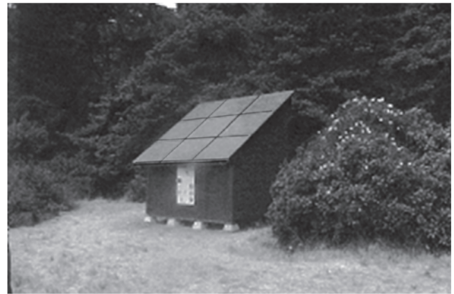
Figure 3-24. Photograph of 960 W PV array at Kirby Cove Campground in California. Deep-cycle batteries, inverter, and balance of system are located in the shed enclosure under the solar panels (Photo by the author).
