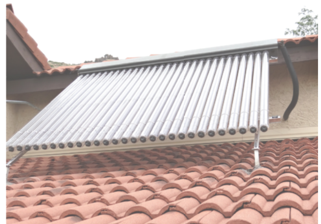
Figure 7-5. Evacuated-tube solar collector for heating domestic hot water at solar home in Golden, Colorado. (Photo by the author)
