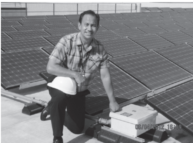
Figure 3-22. Facility manager Larry Barrett inspects the PV system on the roof of the Jerry L. Pettis Memorial VA Medical Center in Loma Linda, California. (Photograph courtesy of Larry Barrett)
