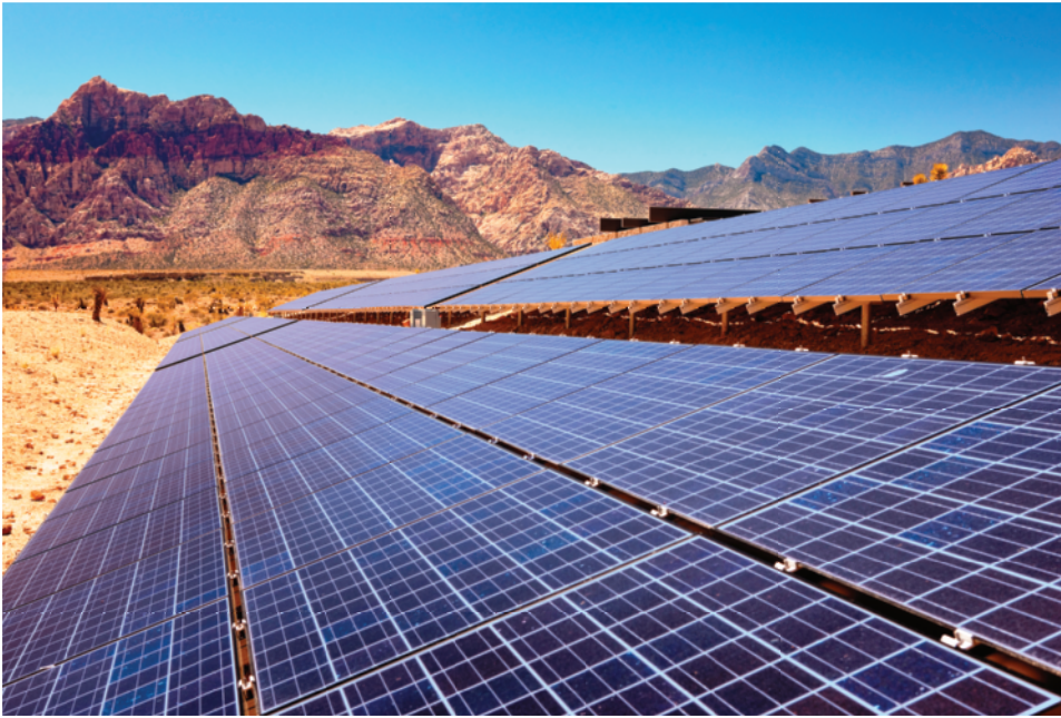
Figure 7-14. Harvesting energy from the sun, the 65-kW STC photovoltaic array provides power to the new Red Rock Canyon Visitor Center, and an interpretive opportunity for visitors. (Photo by Robert Reck, courtesy Line and Space LLC)
