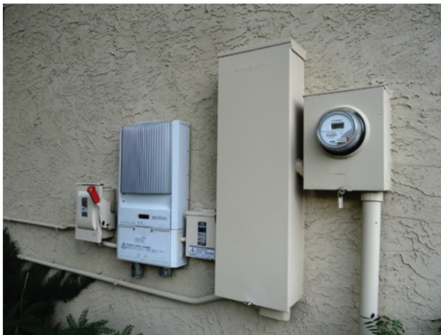
Figure 7-4. Photograph of photovoltaic balance of system components. From left to right: DC disconnect; inverter (2.5 kW, 240 VAC); AC disconnect; utility interconnection in building electrical panel; and bi-directional utility meter. (Photo by the author)
