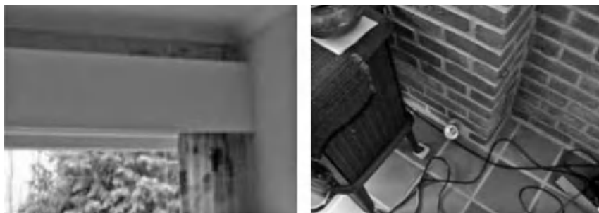
Figure 10.11. Mould on the lintel (on the left) caused by the ventilation pipe connecting the living room to the crawlspace (the pipe is where the lamp sits, see picture on the right).
