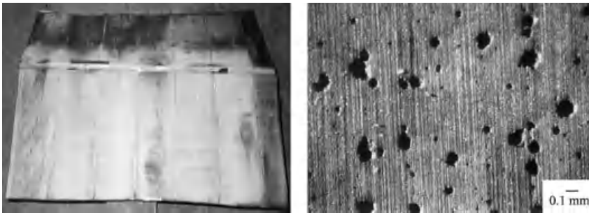
Figure 7.14. Corroded underside of a zinc/titanium cover.
