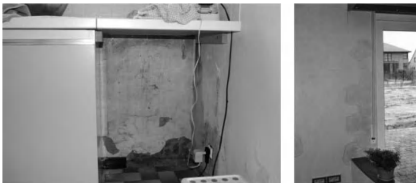
Figure 11.3. Rain penetration: on the left seen as rising damp in the inside, on the right giving a wet inside leaf along window bay.
