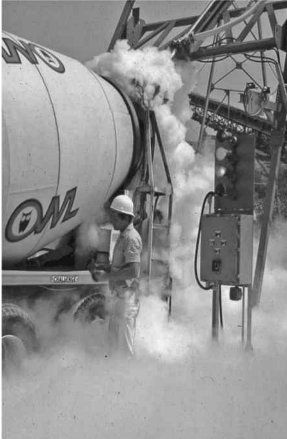
FIGURE 5.42 Using nitrogen for cooling.
