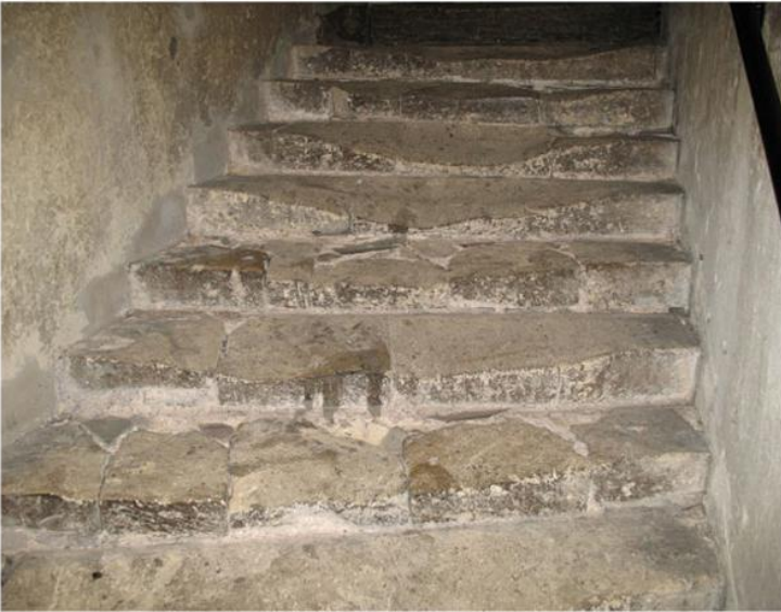
10.15 Worn treads. (Cliveden Conservation)
