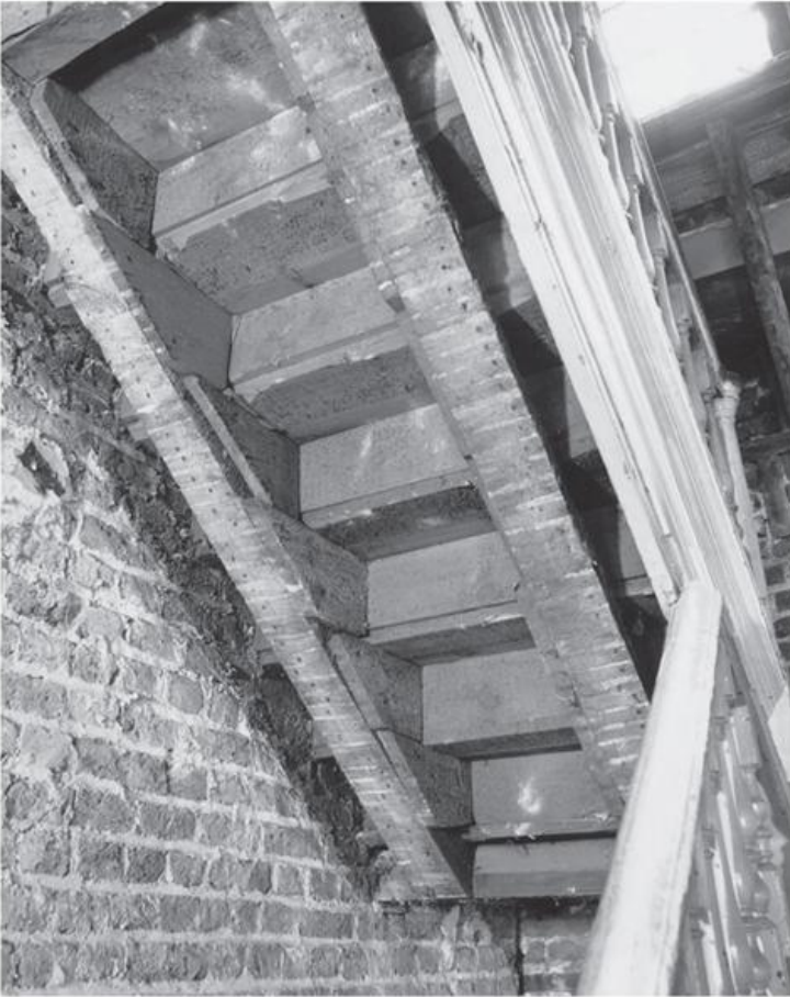
4.3 No. 37 Craven Street, Charing Cross, c. 1730. A view of the underneath of the closed-string staircase with its usual covering removed during a major conservation programme. It shows very well the substantial timber bearers or carriage pieces that support the actual weight of the staircase structure and which are normally hidden from view. (Courtesy of English Heritage)
