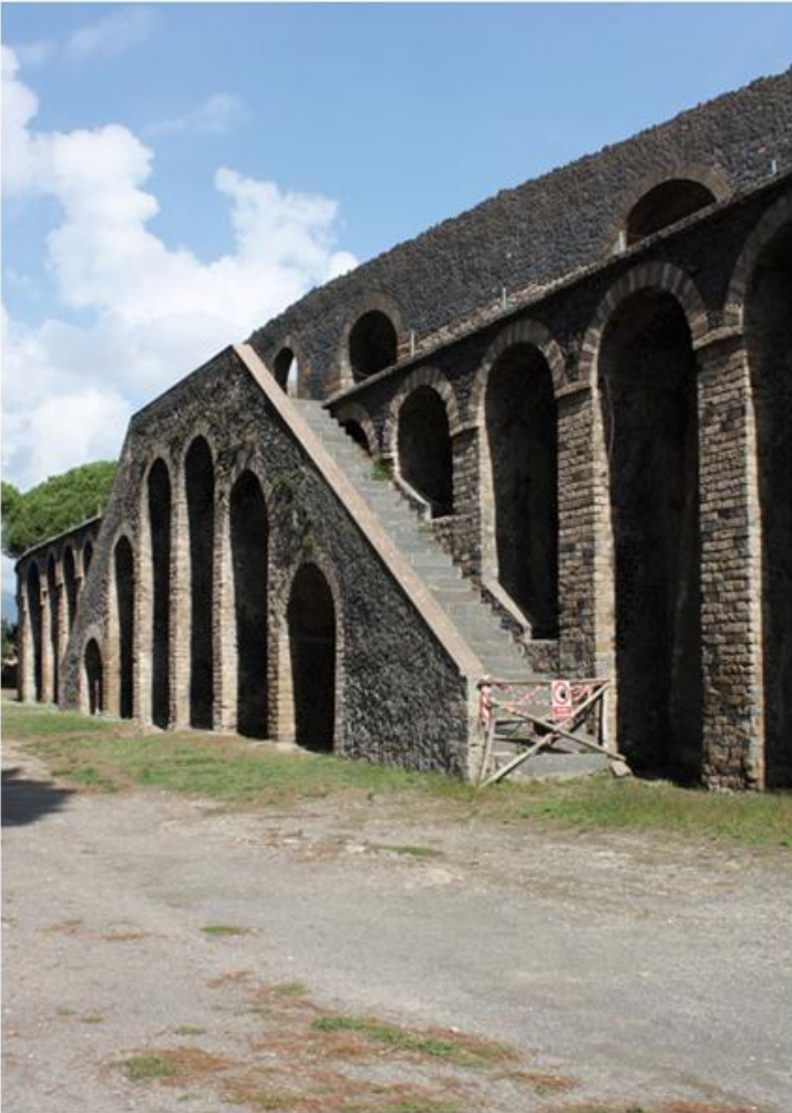
1.18 Pompeii, Italy, the amphitheatre. Double-flight staircases carried on mirrored diminishing arches. There are two such pairs of flights and this is the northern one. At the extreme north and south ends are single flight
