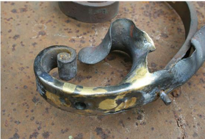
11.8 Repair to a wrought-iron balustrade component. Decorative wrought ironwork subject to severe corrosion
