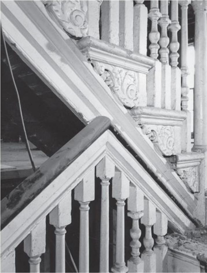
4.2 No. 37 Craven Street, Charing Cross, c. 1730. Detail of the meeting point on a dog-leg staircase of cut-string type. Made of pine, the handrail is stained dark brown to imitate mahogany. While there are three turned balusters per tread they are of the same pattern; however, the turner has had to take into consideration the shrinking of shape to keep the design coherent, hence the
