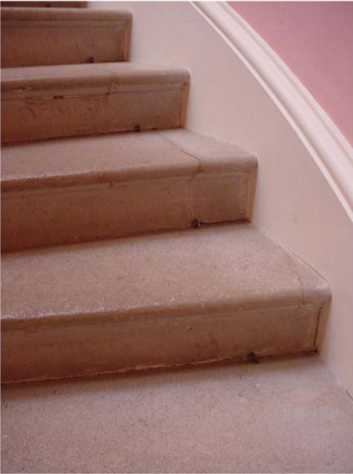
10.8 Structural movement resulting in fractured treads. (Cliveden Conservation)
