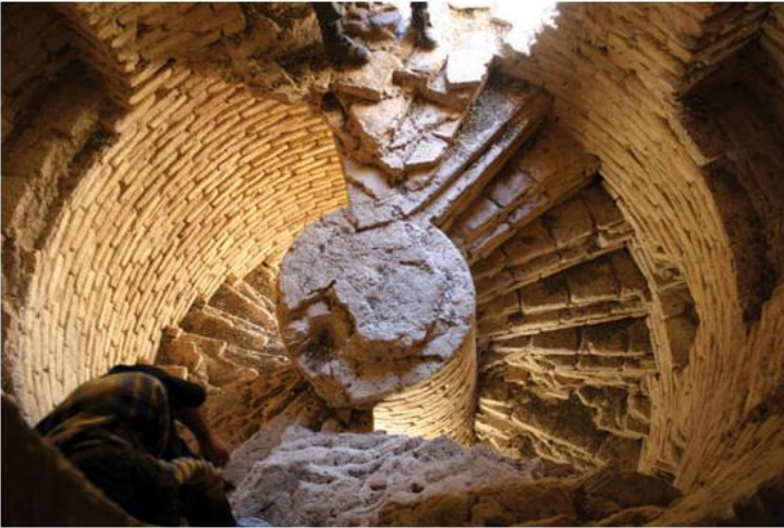
1.24 Jam minaret, western Afghanistan, the two spiral flights clearly visible with a figure (the boots only visible) standing atop one flight while another in the left foreground nears the top of the other flight. Each tread has a rebate at the leading edge where there was once a timber element or nosing. (David Thomas, MJAP 2005)
