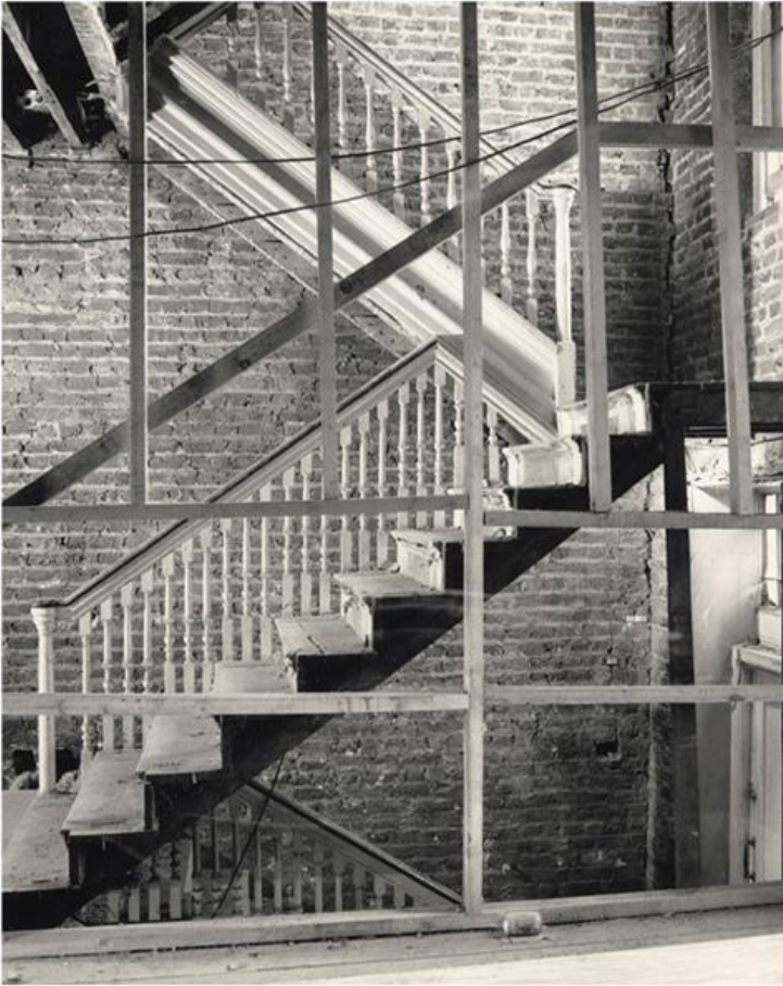
4.1 No. 37 Craven Street, Charing Cross, c. 1730. An unusual view taken during the substantial refurbishment in the late 1980s of almost the whole eastern row of houses. All the wall panelling has been removed thus revealing the usually hidden structure of the staircase from the first to second floor. The difference between a cut and open string stair is clearly illustrated. (Courtesy of English Heritage)
