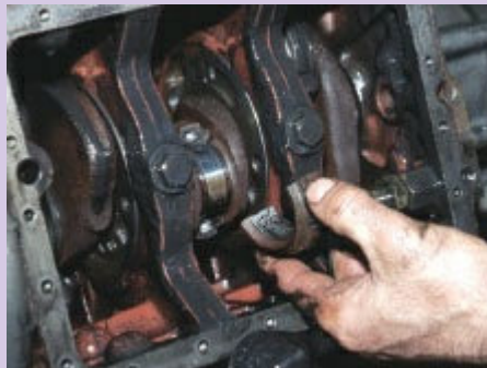
4 Detach and remove the con-rod caps. A light tap on either side with a hammer will loosen them.
