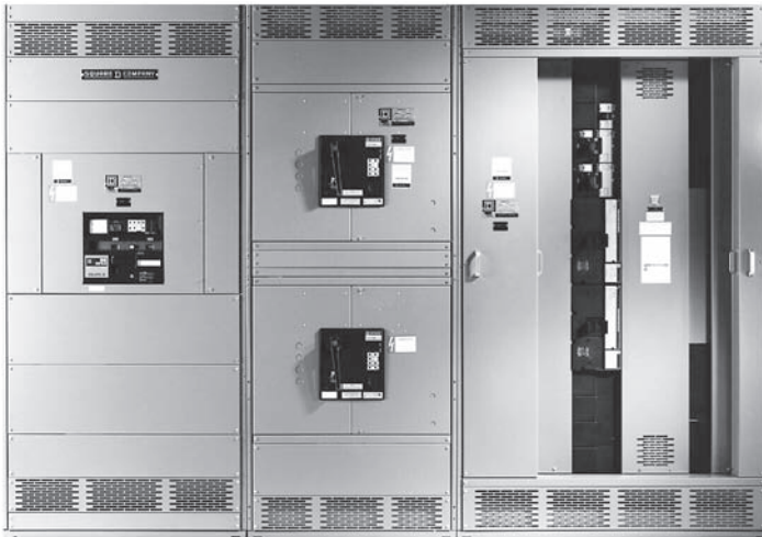
Fig. 4-5 This is a switchboard. Even if positioned against a wall, it is still freestanding equipment. Most, including the one pictured, are capable of rear access. ( Square D Company )
