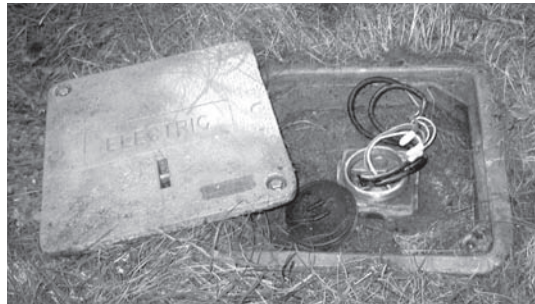
Fig. 27-8 A handhole enclosure, in this case without a bottom, in use. This one is unusual because it encloses another box instead of housing the open wires directly, but under the 2008 NEC it could do so provided both the wires and the splices were listed as suitable for wet locations. In this case the appropriately rated inner box allows for conventional splicing methods.
