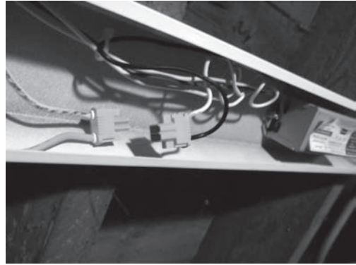
Fig. 29-5 This little disconnect, shown pulled open, opens both sides of the circuit feeding this fluorescent luminaire ballast.
