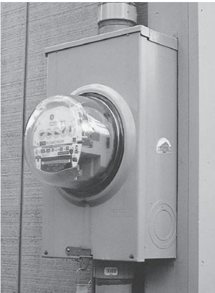
Fig. 16-20 A detachable outdoor meter and the socket in which it is installed. Meters of this type are exposed to the weather.
