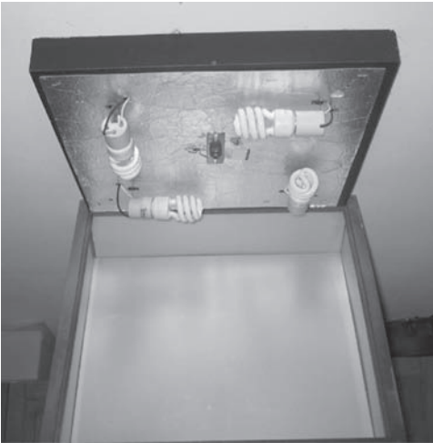
Fig. 14-11 Incandescent luminaire retrofitted with self-ballasted compact fluorescent lamps, decreasing energy consumption by 77%.
