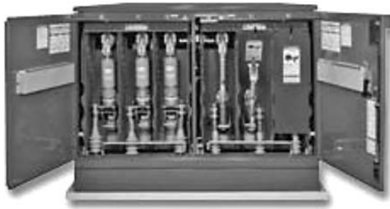
FIGURE 4.11 Pad-mount substation with fuses (livefront).
