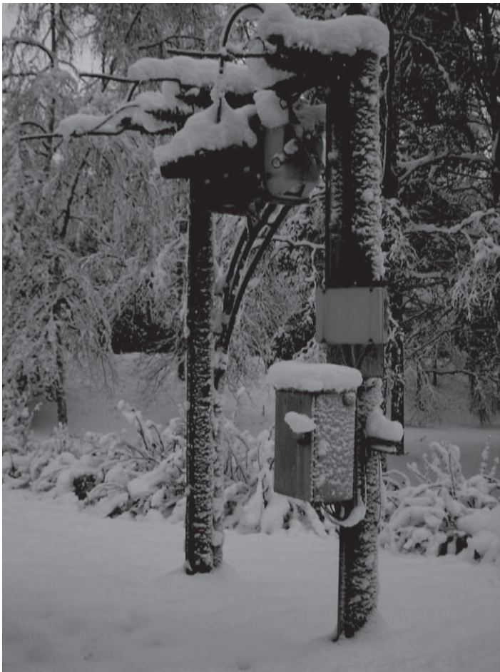
FIGURE 4.14 Overhead customer substation showing transformer and, at the pole top, an ice-encrusted air break switch.
