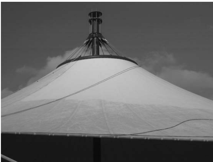
12.62 Results of cleaning membrane (CC Almenara, Lorca. BAT, Spain).
