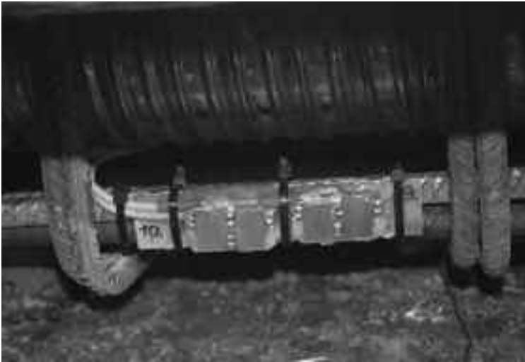
9.6 The ER probes installation on-site on a bottom side of bridge tendon before concreting (Črni kal viaduct).
