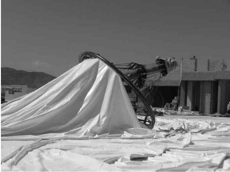
12.57 Preparing the membrane and connection with the structure (CC Almenara, Lorca. BAT, Spain).
