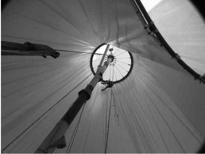
12.60 Stabilization of central mast during lifting process (CC Almenara, Lorca. BAT, Spain).
