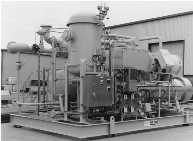
Figure 19.4 Purpose built package for R125 cooling using R410A refrigerant (J&E Hall)
