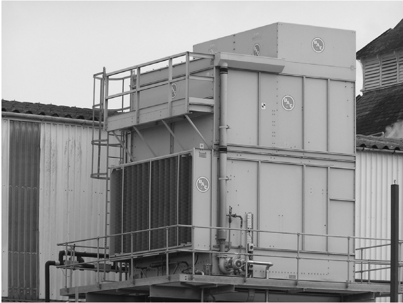
Figure 6.8 Evaporative condenser installation (Baltimore Aircoil)
