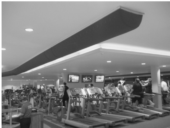
Figure 24.19 Textile ducting providing air distribution in a gymnasium (Business Edge)
