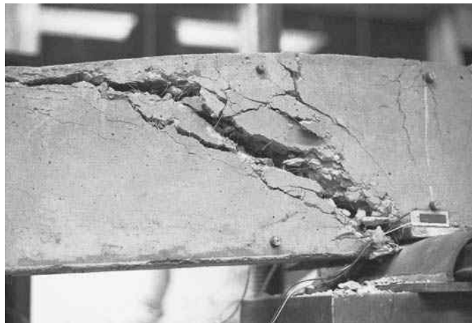
Shear failure near a middle support.
