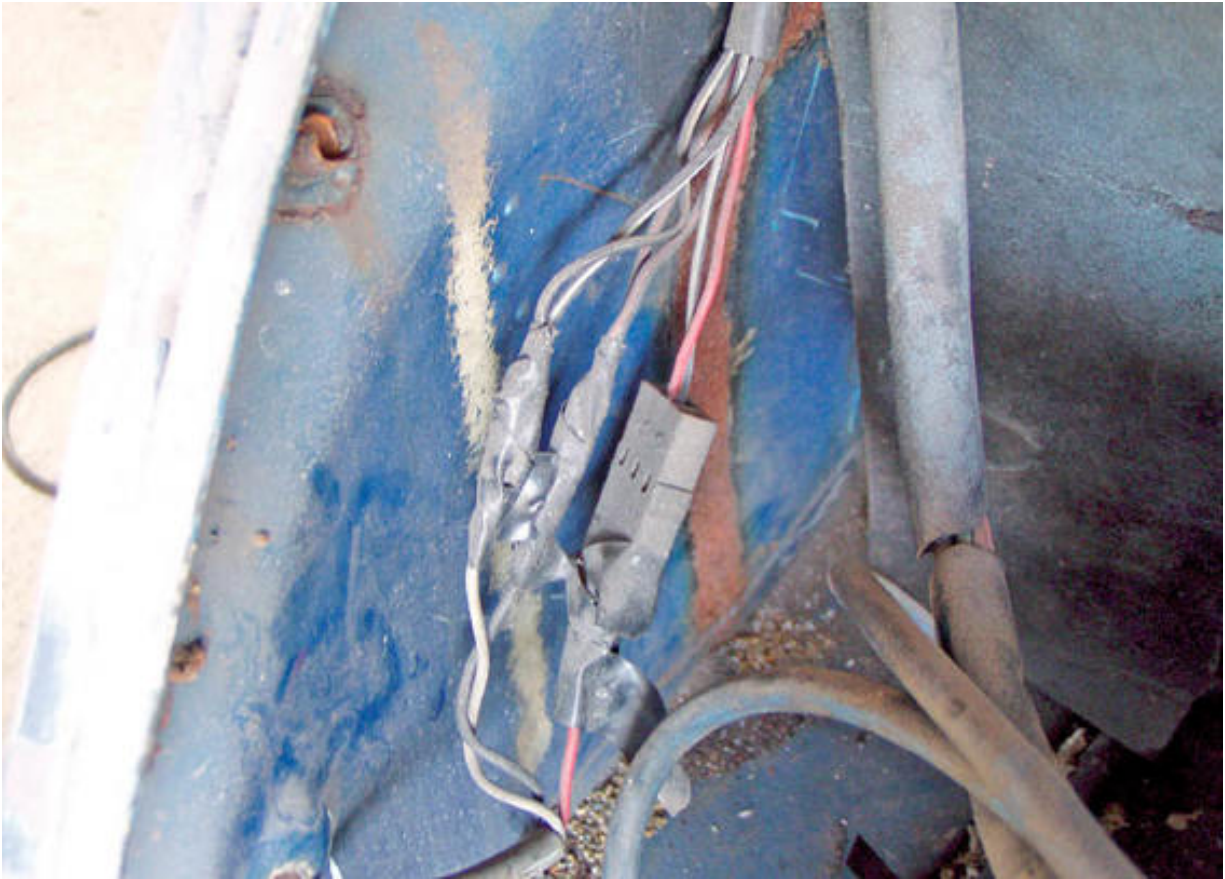
Typical wiring - untidy taped joints, but at least it is colour-coded.
