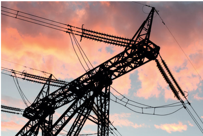
Figure 6.2 The electricity grid power supply mostly travels along conductors supported by pylons.
