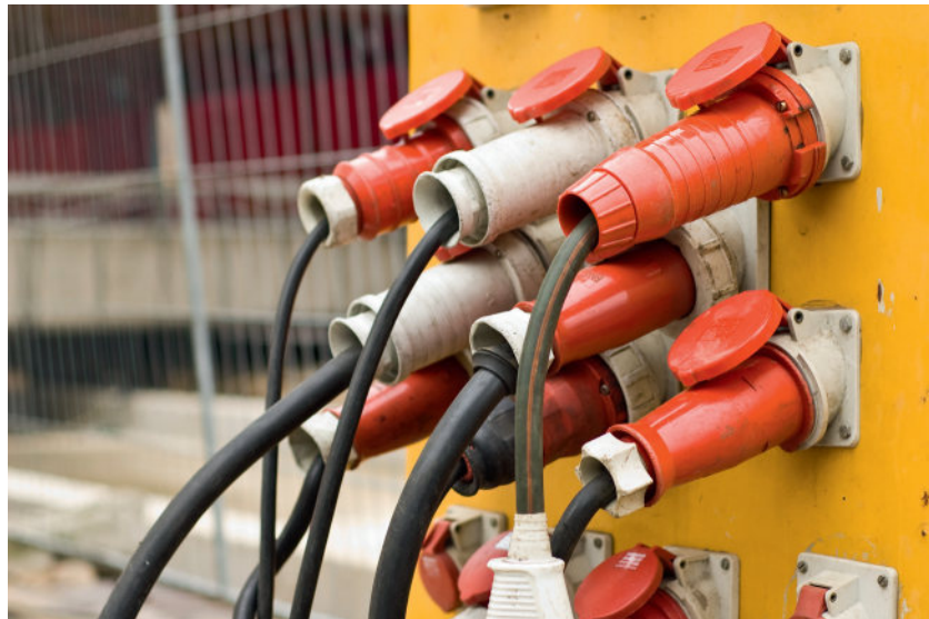
Figure 4.27 Temporary electrical supply.
