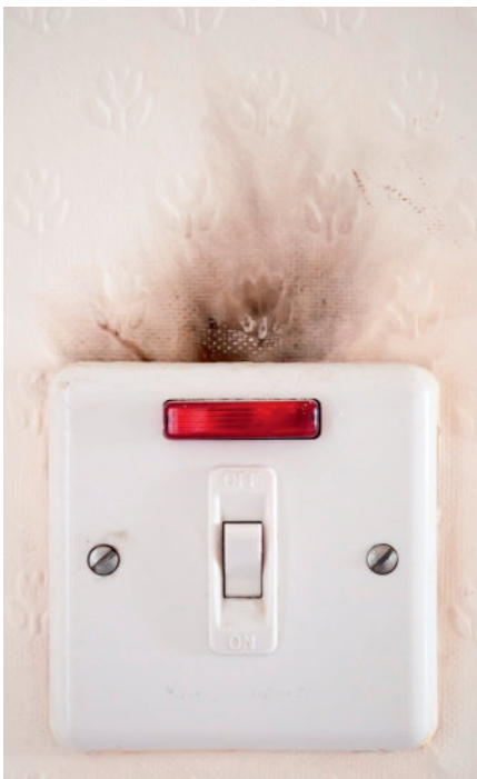
Figure 5.3 Clearly an electrical fault is hiding behind this switch plate.
