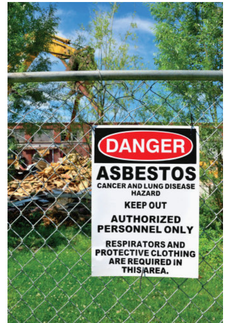
Figure 1.33 Hazardous areas should be clearly signposted.
