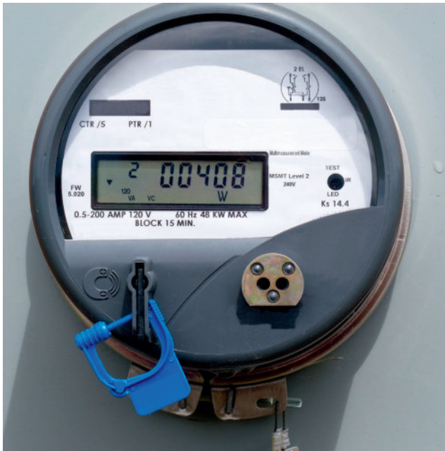
Figure 2.2 Smart electricity meter.
