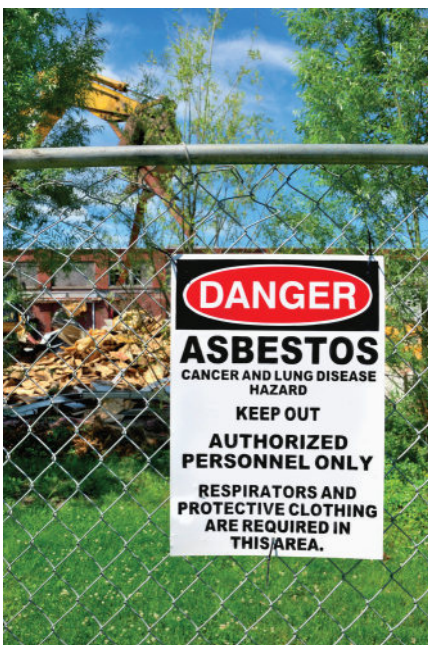
Figure 4.34 Asbestos warning sign.
