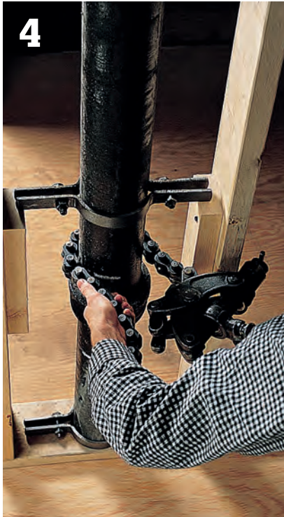
4 Wrap the chain of the snap cutter around the pipe, so that the cutting wheels are against the chalkline.
