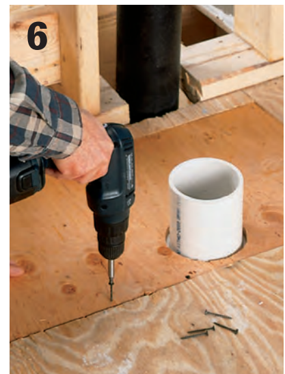
6 Cut a piece of exterior-grade plywood to fit the cutout floor area, and use a jigsaw to cut an opening for the toilet drain stub-out. Position the plywood, and attach it to joists and blocking with 2" screws.
