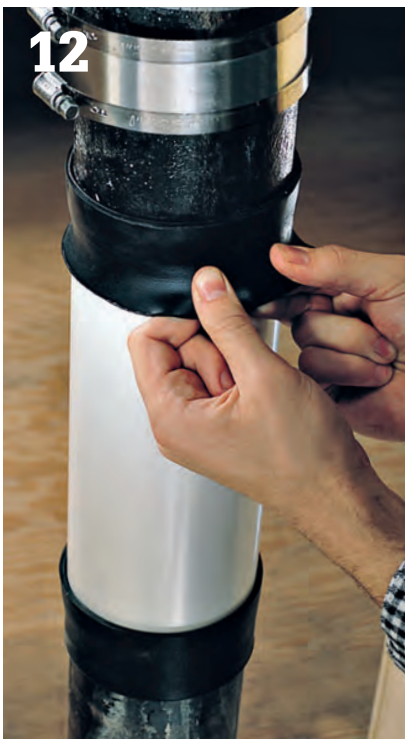
12 Roll the ends of the neoprene sleeves over the ends of the new plastic pipe.
