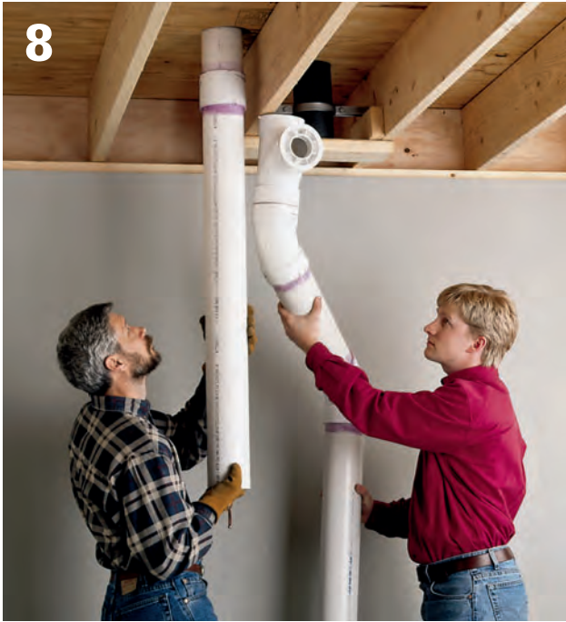
8 Cut a PVC plastic pipe to length, raise it into the opening, and dry-fit it to the T-fitting. Note: For very long pipe runs, you may need to construct this vertical run by solvent-gluing two or more segments of pipe together with couplings.
