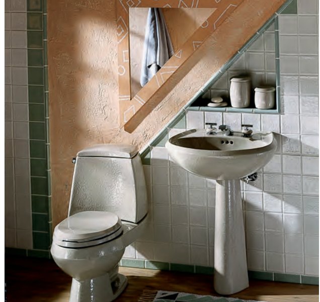
In this half bath, the toilet and sink are close to the main stack for ease of installation, but are spaced far enough apart to meet minimum allowed distances between fixtures. Check your local code for any restrictions in your area. Generally, there should be at least 15" from the center of the toilet drain to a side wall or fixture, and a minimum of 21" of space between the front edge of the toilet and the wall.
