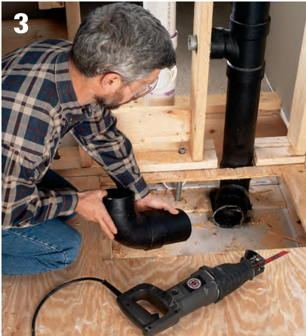
3 Cut away the old closet bend as close as possible to the old waste-vent stack, using a reciprocating saw with metal-cutting blade, or a cast iron cutter.
