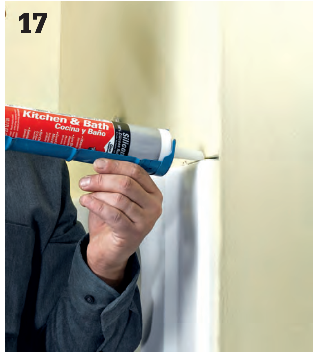
17 Finish the walls and then caulk between the enclosure panels and the wallcoverings with silicone caulk.
