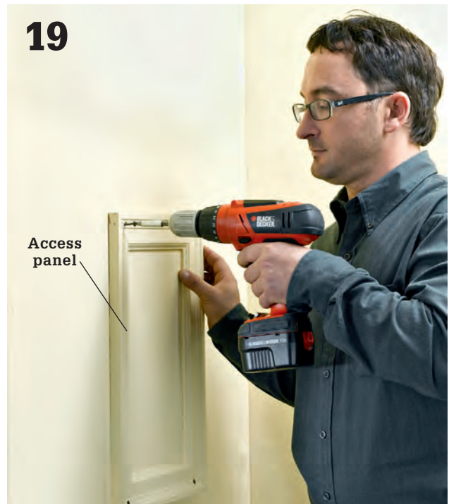
19 Make an access panel and attach it at the framed opening created in step 8. A piece of \frac{1}{4} " plywood framed with mitered case molding and painted to match the wall is one idea for access panel covers.
