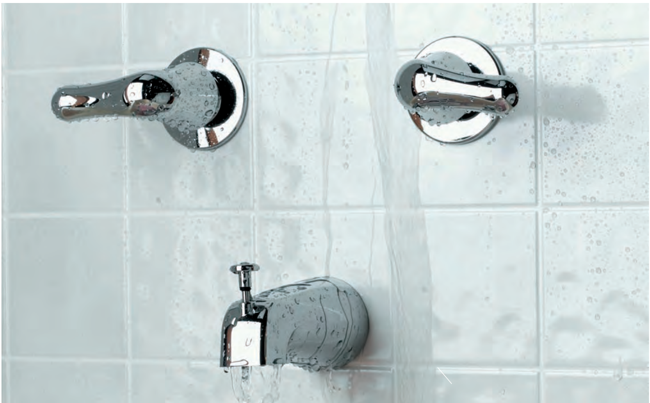
Tub/shower plumbing is notorious for developing drips from the tub spout and the showerhead. In most cases, the leak can be traced to the valves controlled by the faucet handles.
