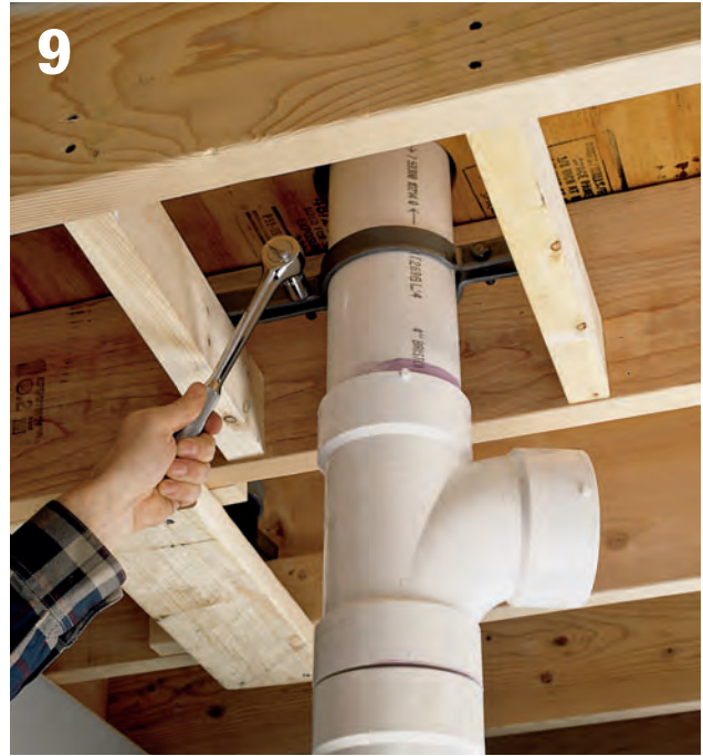
9 Check the length of the stack, then solvent-glue all fittings together. Support the new stack with a riser clamp resting on blocks attached between basement ceiling joists.
