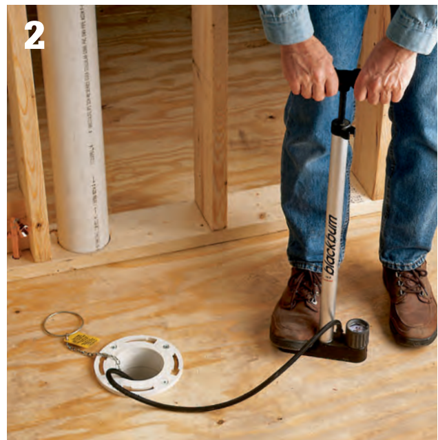
Block toilet drains with a test balloon designed for a closet bend. Large test balloons may have to be inflated with an air pump.
