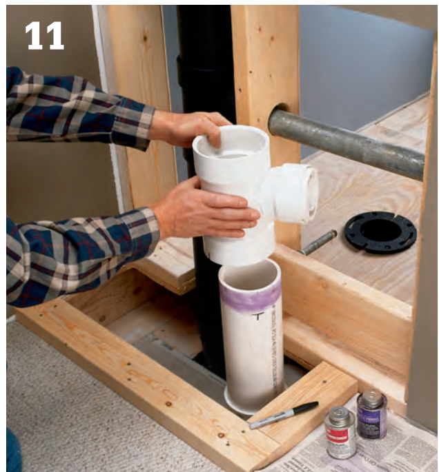
11 Add additional lengths of pipe, with waste T-fittings installed where other fixtures will drain into the stack. In our example, a waste-T with a \frac{1}{2} " bushing insert was installed where the vanity sink drain was attached to the stack. Make sure the T-fittings are positioned to allow for the correct downward pitch of the branch drains.
