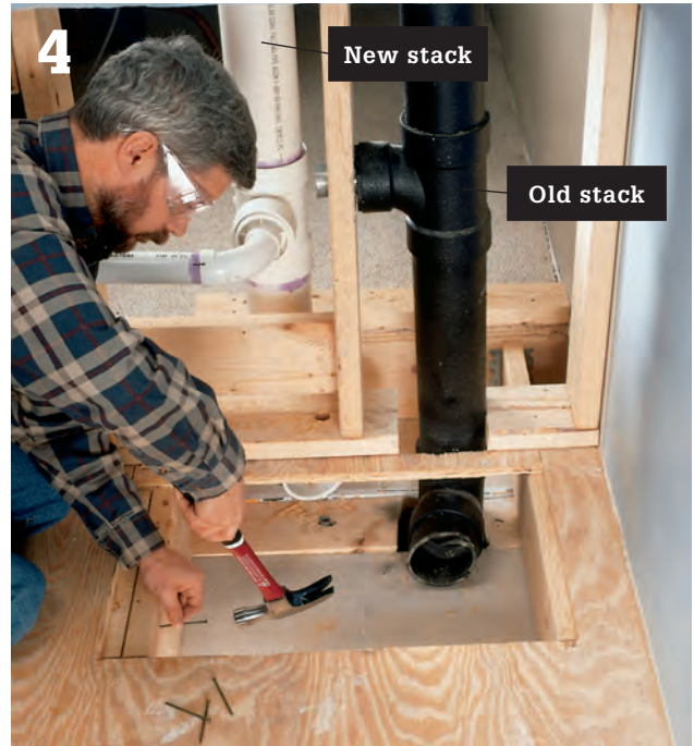
4 If a joist obstructs the route to a new waste-vent stack, cut away a section of the floor joist. Install double headers and metal joist hangers to support the ends of the cut joist.
