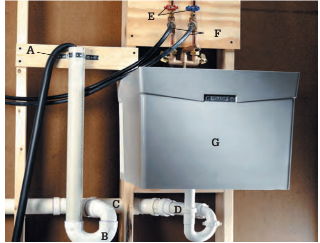
A washing machine with standpipe drain: washing machine drain hose (A), 2" standpipe with trap (B), waste line (C), utility sink drain pipe (D), hot and cold supply lines with hose bibs (E), rubber supply hoses to washing machine (F), and utility sink (G).
