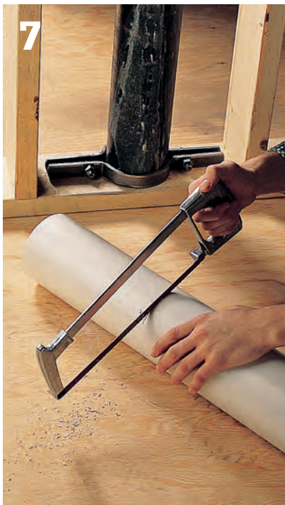
7 Cut a length of PVC plastic pipe to be 1/2" shorter than the section of cast-iron pipe that has been cut away.
