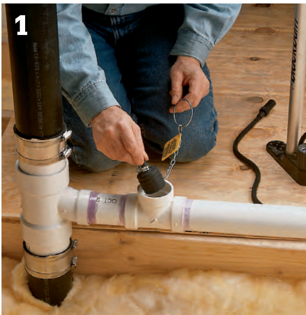
Insert a test balloon into the test T-fittings at the top and bottom of the new DWV line, blocking the pipes entirely. Note: Ordinary T-fittings installed near the bottom of the drain line and near the top of the vent line are generally used for test fittings.
