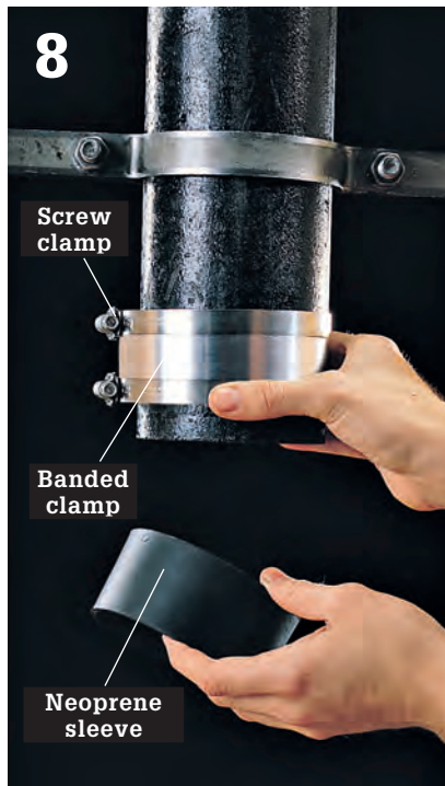
8 Slip a banded coupling and a neoprene sleeve onto each end of the cast-iron pipe.
