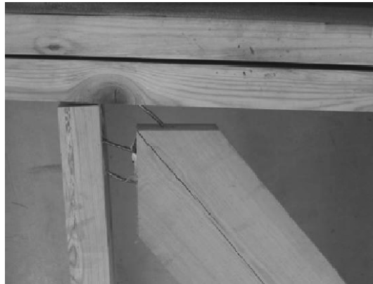
Figure 8.10. Rupture of the joint of the stressed strut at the foot of the fifth upright
