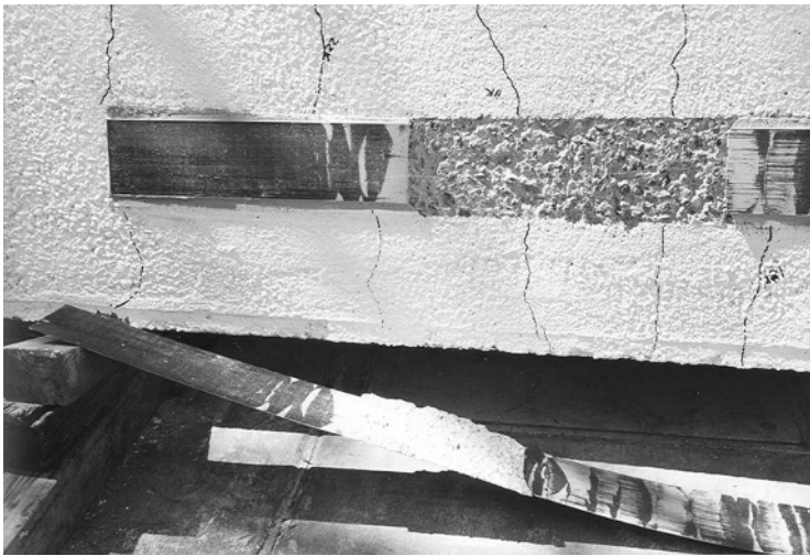
5.4 Close-up showing splitting within the prefabricated strip.
