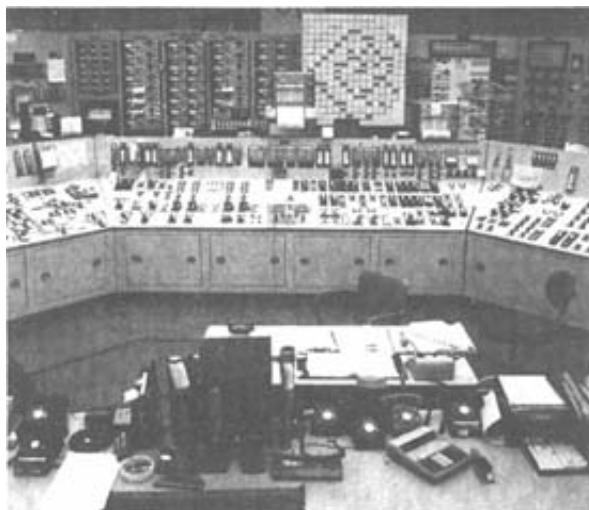
Figure A21.2 Control room at TMI 2 (Kemeny, 1979)
