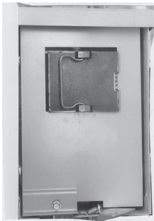
► Figure 6-7 Disconnect switch used for air conditioning equipment. (Source: Delmar/Cengage Learning)
