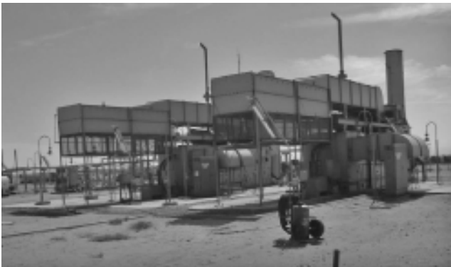
FIGURE 4.2 Gas turbine generator.
