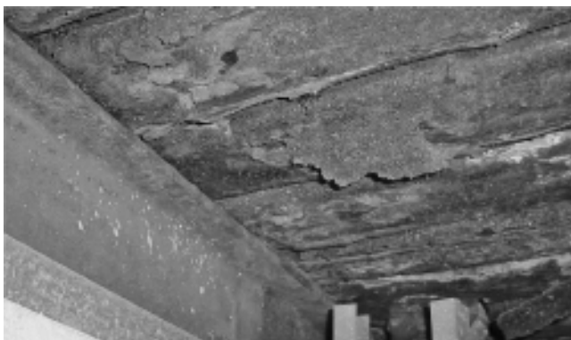
FIGURE 8.12 Corrosion in a corrugated sheet.
