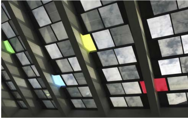
Figure 10.8 Semitransparent colored amorphous silicon thin-film photovoltaic glazing. Courtesy of Onyx Solar Group llc.
