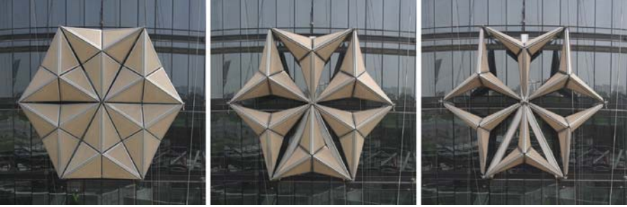
Figure 8.21 Al Bahar Towers facade operation. Courtesy of Arup.
