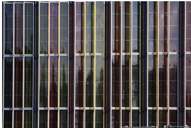
Figure 10.17 SwissTech Congress Center DSSC facade. Courtesy of Solaronix SA.
