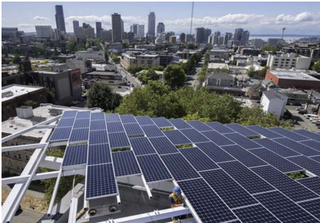
Figure 1.15 Bullitt Center, photovoltaic roof. Courtesy of John Stamets/Bullitt Foundation ©.
