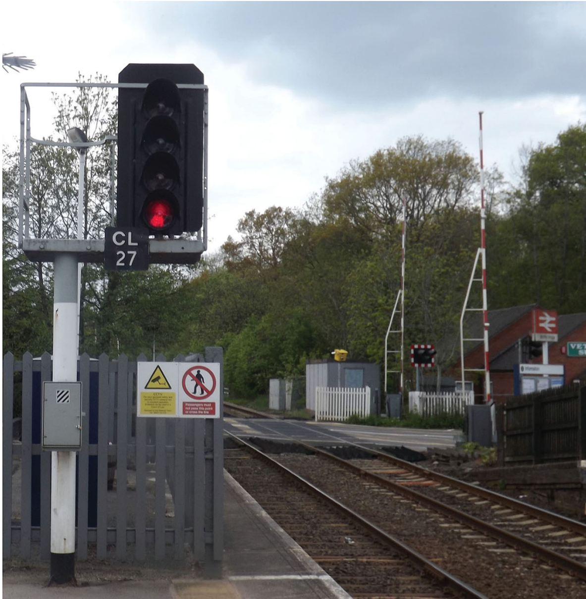
A modern four-aspect signal located on the platform at Blythe Bridge Station, Staffordshire.
