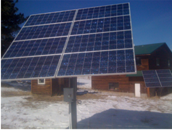
Figure 2.5. Residential PV system.
