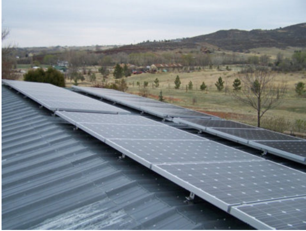
Figure 9.7. Metal roof flush-mounted PV array.
