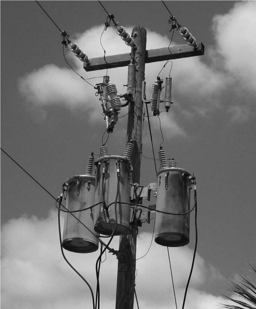
Figure 1.6 A bank of service transformers does not look new, because they aren't, but they are good to go in a system that is trying to get the most from its past investments in equipment. The utility's challenge is to separate these units, which can be expected to give satisfactory service for many years to come, from other units that won't.
