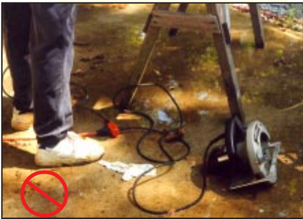
Combinations of hazards increase risk.
