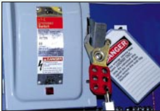
Always lock out and tag out circuits.
