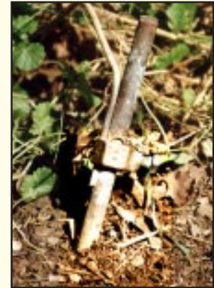
Grounding rod in the earth.
