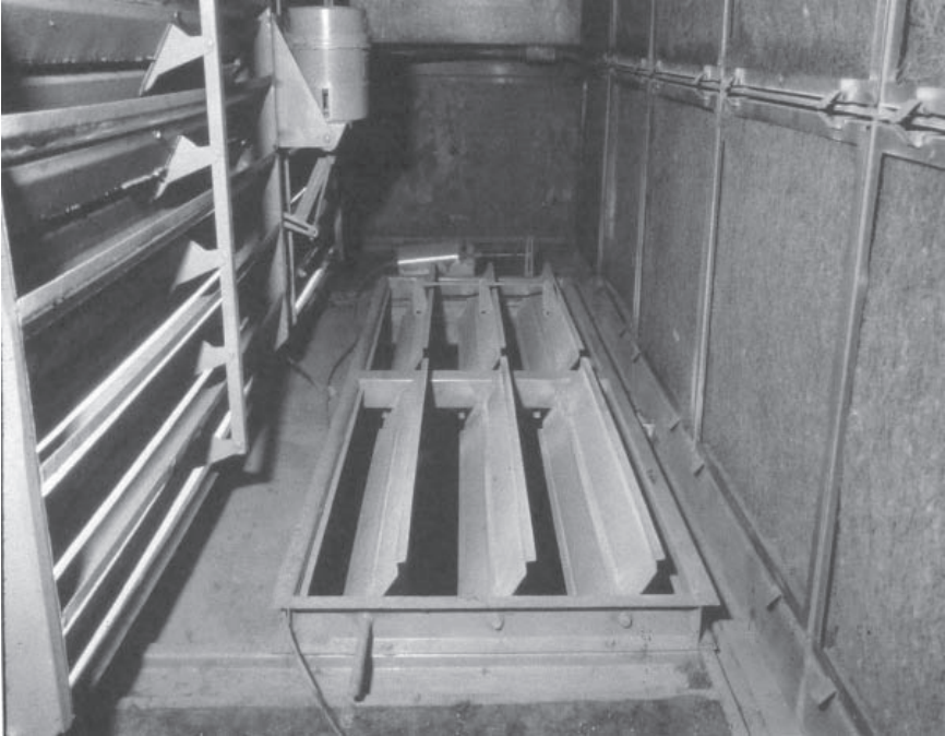
Figure 8-14. Parallel blade dampers in mixed air plenum. Notice blade action for opposed blade and parallel blade dampers.
