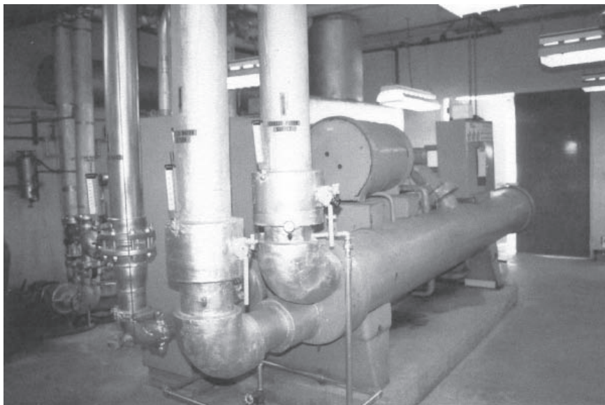
Figure 6-1. Centrifugal Mechanical Chiller
