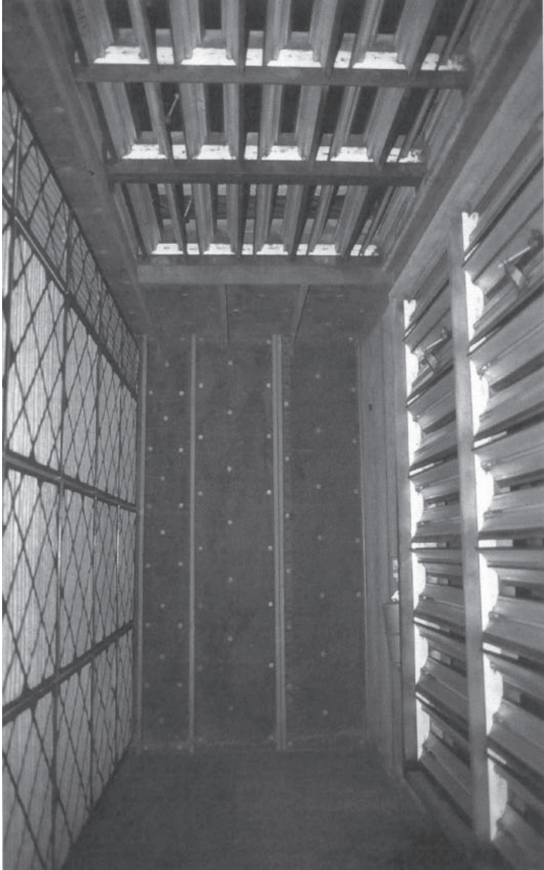
Figure 8-13. Opposed blade dampers in mixed air plenum. Notice blade action for opposed blade and parallel blade dampers.
