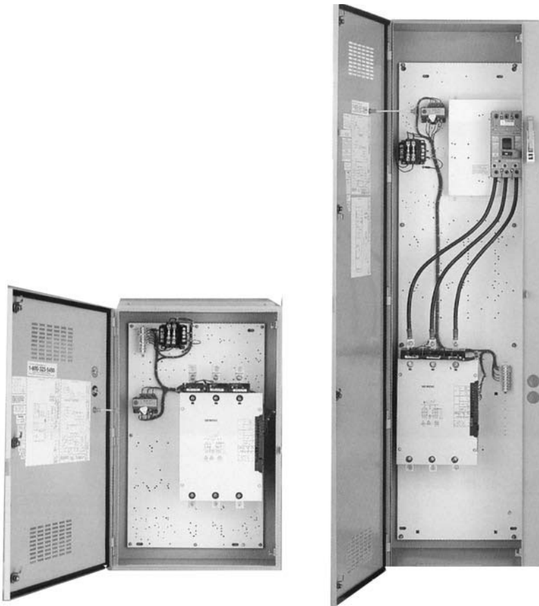
Figure 16-2 Solid-state motor controllers mounted in cabinets. (Courtesy of Benshaw, Inc.)
