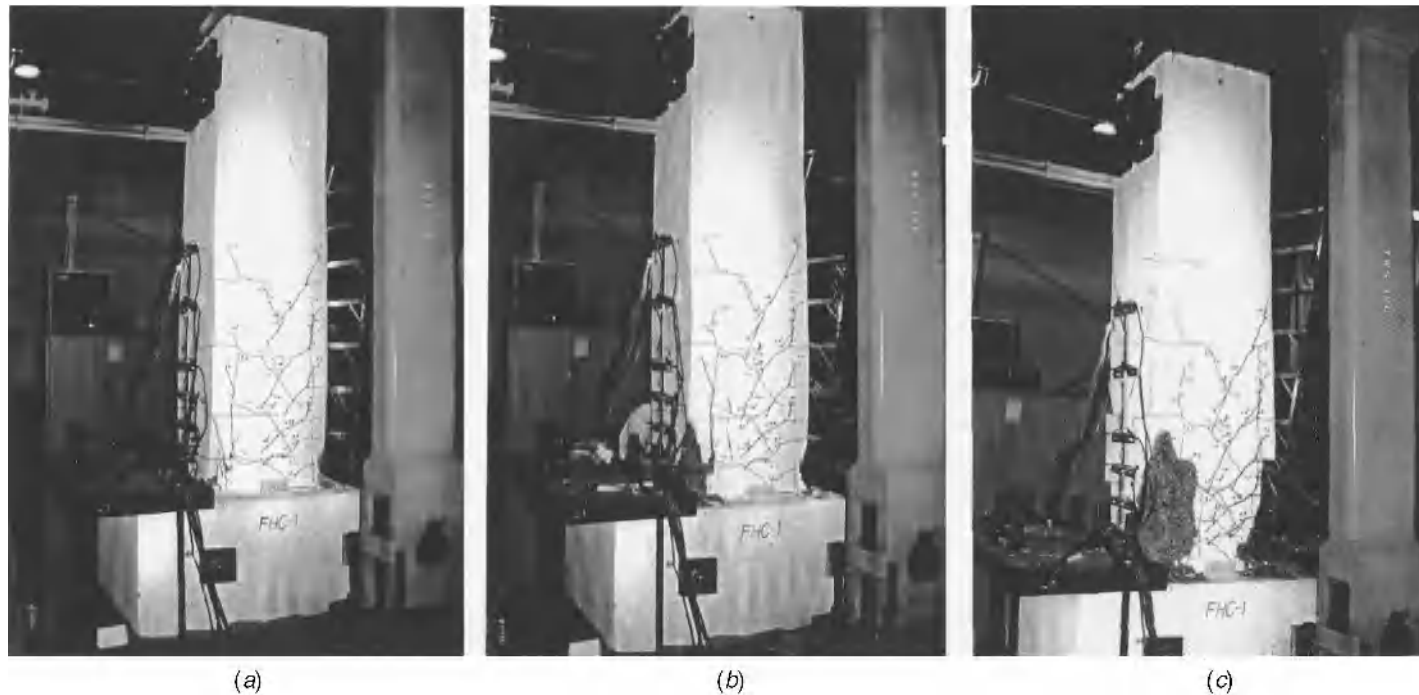
Figure 2.2.7 Crack patterns for Specimen 1 at various loading stages. (a) At \delta/h_x = 2.0\% . (b) At drift ratio \delta/h_x = 3.0\% . (c) At \delta/h_x = 6.0\% .
