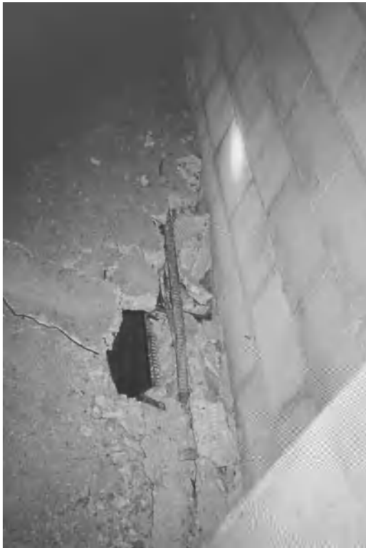
Figure 3.3.5 Buckling of chord bars in a diaphragm.
