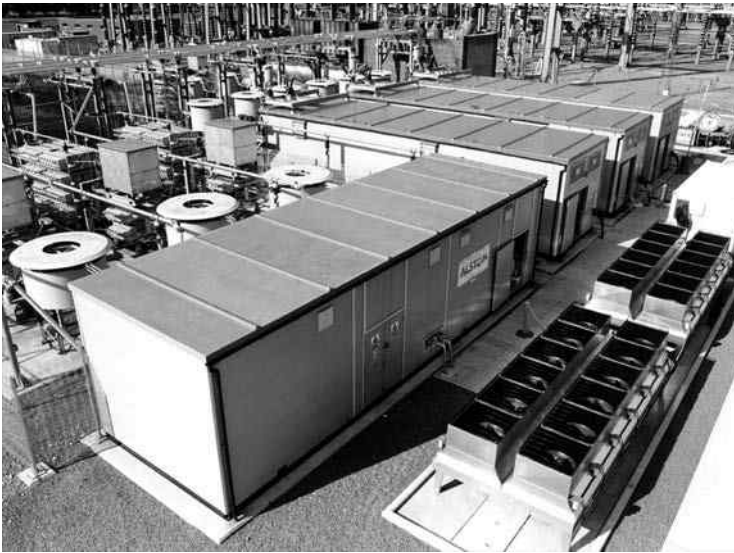
Figure 4.22 View of 225 MVA STATCOM
