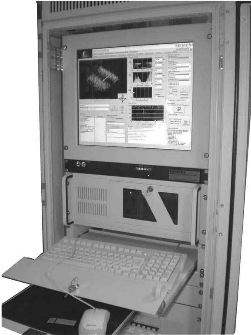
Figure 21.30 ISCM control cubicle showing PDM diagnostics display
