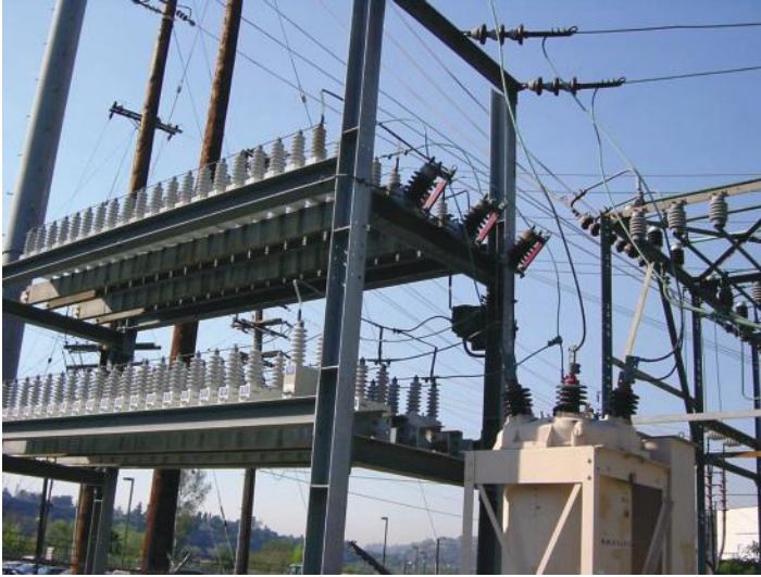
FIGURE 2.25 Substation capacitor racks.
