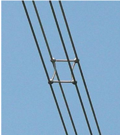
FIGURE 6.17 Bundled conductor with four subconductors.
