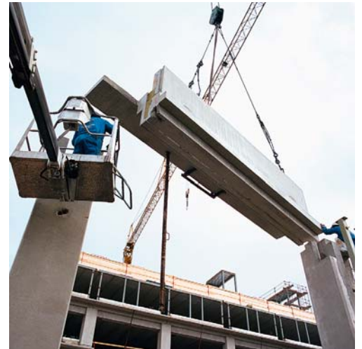
Top: Installing precast floor plank Bottom: Edge beam with cantilever ledge being lifted onto column heads
