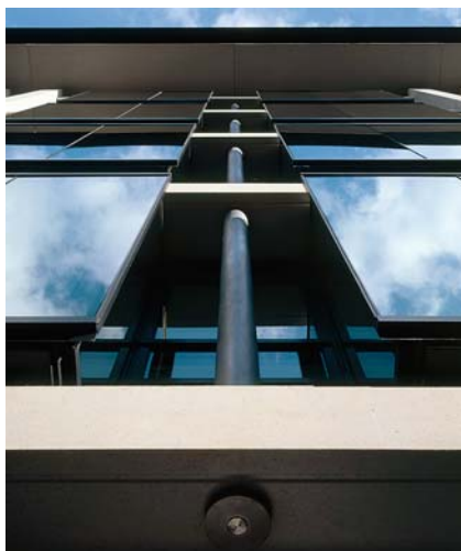
Left: End elevation on East Street Right: Window box proud of precast facade
