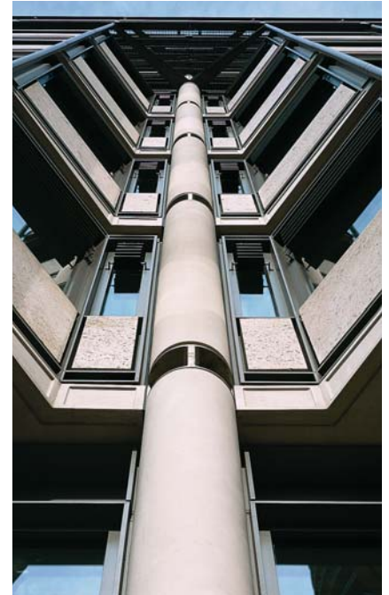
The GRC pilasters and bay window reveals combine with flat ashlar panels
