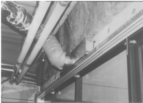
Figure 2-25 Poor inlet duct connection to a supply air ceiling diffuser. The winding flex duct path causes excessive air turbulence and noise at the diffuser's inlet collar. This diffuser could produce noise levels as much as 15 dB higher than the manufacturer's catalog data.
