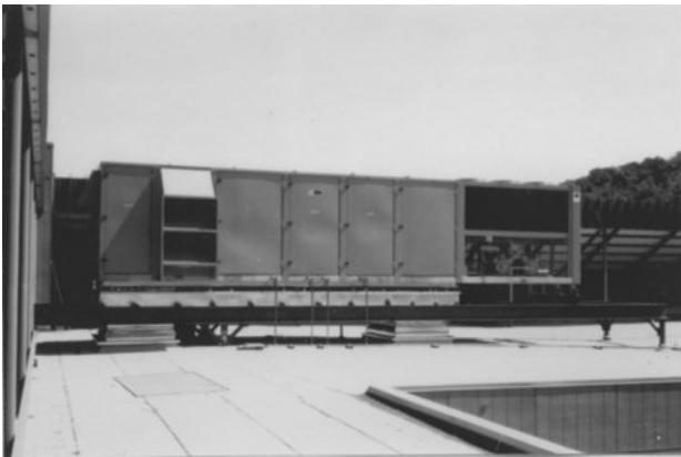
Figure 8-6 Excellent rooftop package unit installation; the unit is resting on spring isolators and an elevated frame, thereby avoiding contact with the roof.
