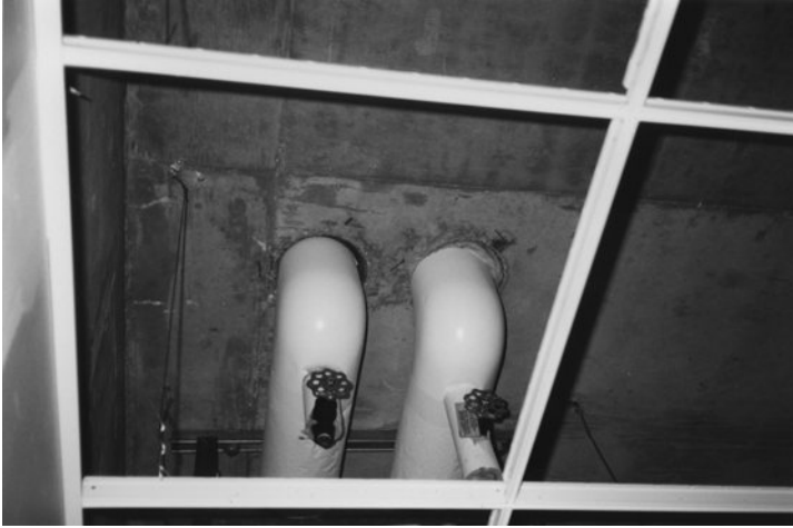
Figure 8-21 View of pipe penetration from below roof. The pipe on the right is contacting the left edge of its penetration. This installation allowed pipe vibration to excite the roof slab, which radiated the energy as noise.
