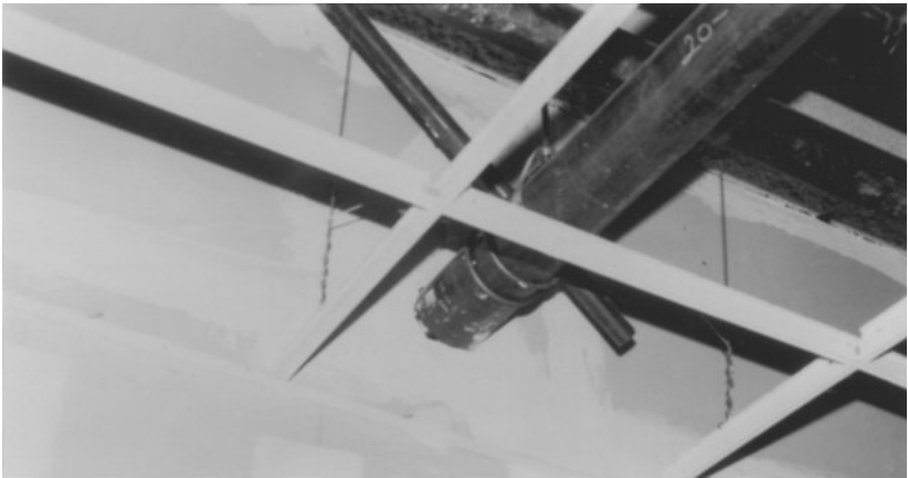
Figure 8-22 Non-isolated pipe penetration. Rigid contact allows pipe vibration to enter the wall, which radiates the energy as noise.
