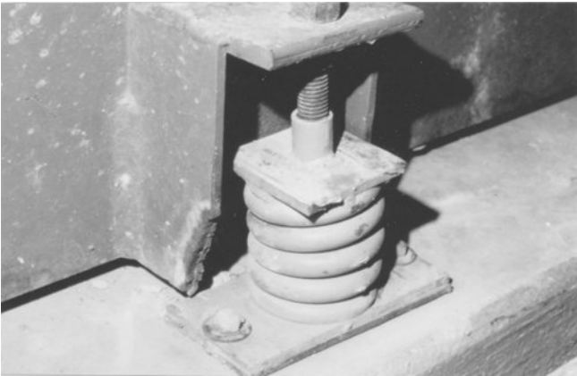
Figure 7-6 Overloaded free-standing floor mount. The overloading allowed the gussets welded to the side of the equipment frame to rest on top of the isolator baseplate. The lower right corner of the gusset was burned off to eliminate the gusset/baseplate contact. The proper action would have been to replace the overloaded spring with a stiffer one able to carry the heavy load.
