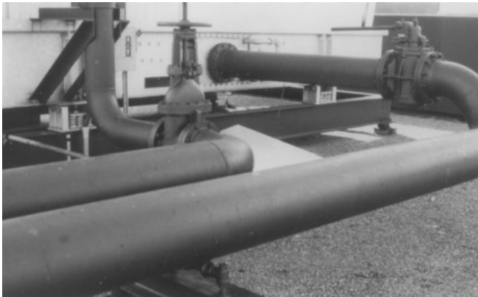
Figure 8-18 Incomplete vibration isolation at cooling tower. Even though the tower is isolated, the condenser water pipe supports are mounted rigidly to the roof. This allows some tower vibration to enter the roof structure.
