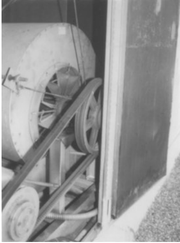
Figure 8-5 View into the fan section of a rooftop unit; the tight cabinet clearance and airflow obstructions at the fan inlet cause excessive turbulence, pressure drop, and noise.
