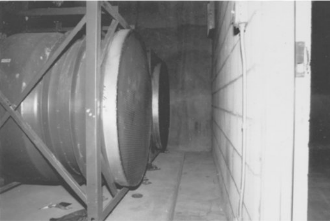
Figure 8-12 Vane-axial fan intakes too close to wall. Airflow through the restricted area between the fans and the wall causes turbulence, surging, and rumble.
