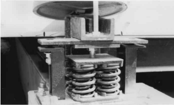
Figure 8-15 Proper installation of a large equipment isolator with stanchion restraints. Note that the springs are centered between the stanchions and are properly compressed and that the equipment mounting plate is floating about 6 mm above the stanchion top plates.
