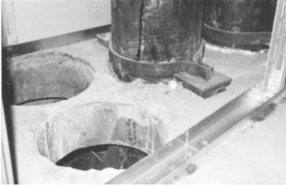
Figure 3-16 Vibration isolation for piping riser. The use of neoprene pads under the steel load-distributing plates indicates that the nearby occupancy was not very noise-sensitive. For more critical cases, steel spring isolators would be used.
