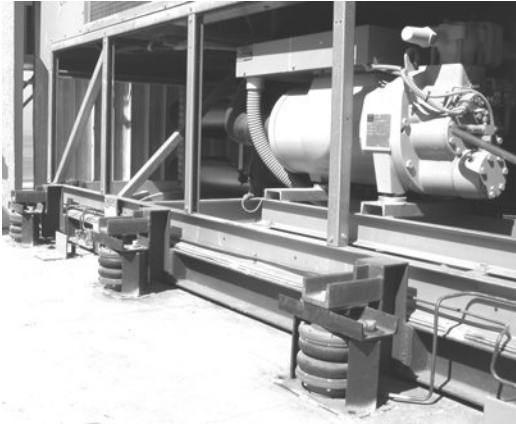
Figure 5-7 Pneumatic isolators (“air bags”) supporting a rooftop air-cooled chiller. Thin metal tubing connects 700 kPa compressed air to each isolator.
