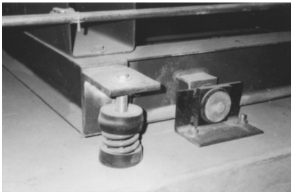
Figure 5-12 Floor mount spring isolator under a height-saving bracket with a separate seismic restraint.
