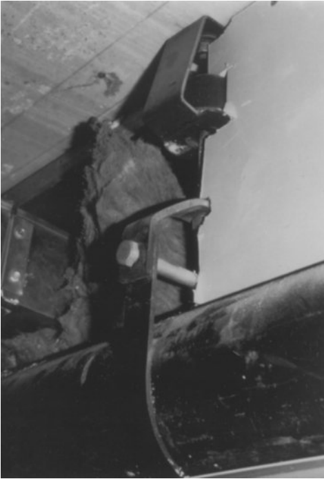
Figure 8-23 Improperly placed neoprene hanger. The drywall assembly forms a vibration transmission bridge across the isolator. This type of interference can be identified and corrected in pre-construction coordination meetings.
