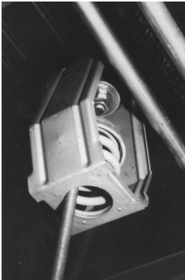
Figure 7-8 Faulty spring hanger installation with hanger rod touching the hanger box. This allows pipe vibration to bypass the spring and enter the building structure above.
