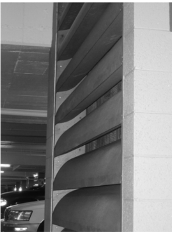
Figure 2-49 Acoustical louver in a parking garage ventilation shaft.
