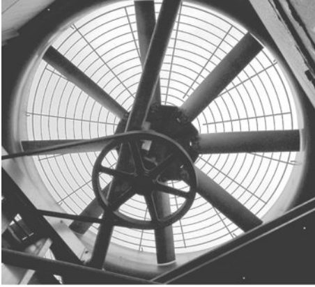
Figure 3-5 View of “standard” cooling tower induced-draft fan.
