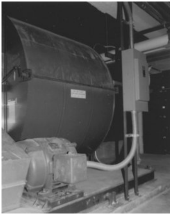
Figure 8-20 Correctly installed flexible conduit between electrical disconnect and motor. The flexible installation reduces fan and motor vibration in the floor slab.
