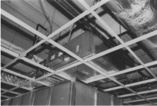
Figure 8-7 Improperly installed fan-powered variable-air-volume unit. The unit is resting on the ceiling grid. This allows unit vibration to transmit directly into the partition below. The partition then acts as a sounding board, radiating noise into the occupied space.
