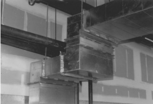
Figure 8-10 Closely spaced rectangular duct fittings produce turbulence and noise. A better offset around the pipes could have been made with a duct section on a 45° slope between the vertical and horizontal sections.
