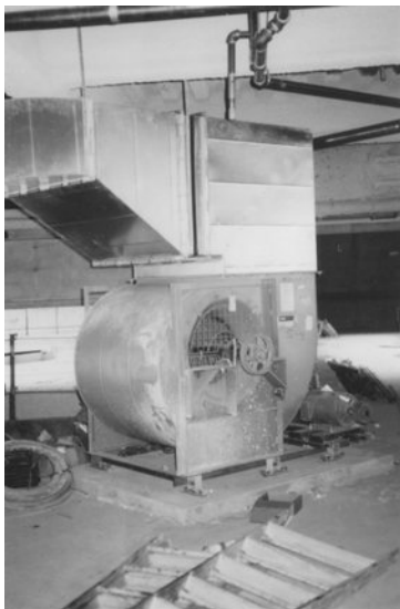
Figure 8-2 Example of poor fan discharge duct design. The mitered elbow with turning vanes and steep transition downstream of the fan outlet cause fan instability and accompanying noise and rumble. A better installation would have used a horizontal discharge fan with fewer downstream fittings.
