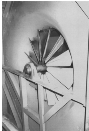
Figure 2-51 Nested inlet vanes obstruct airflow.
