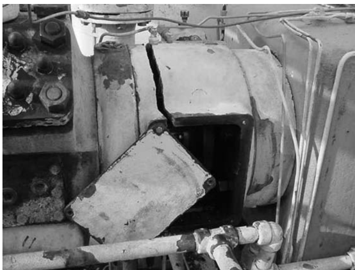
Figure 11-15. Reciprocating Compressor Showing Failed Distance Piece.
