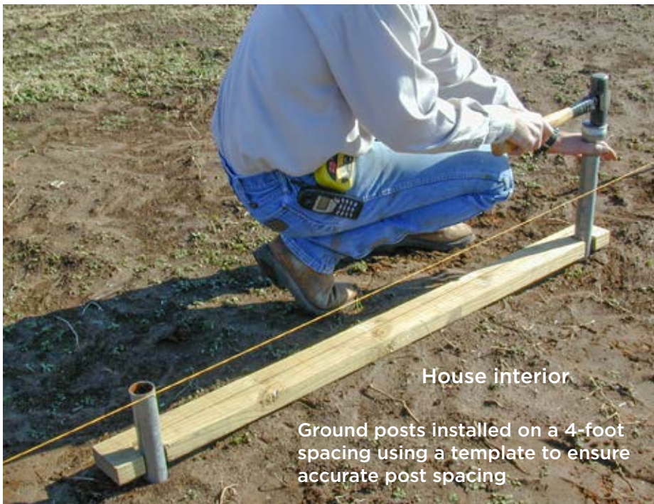
Accurate ground post installation minimizes complications that can arise during house construction.
