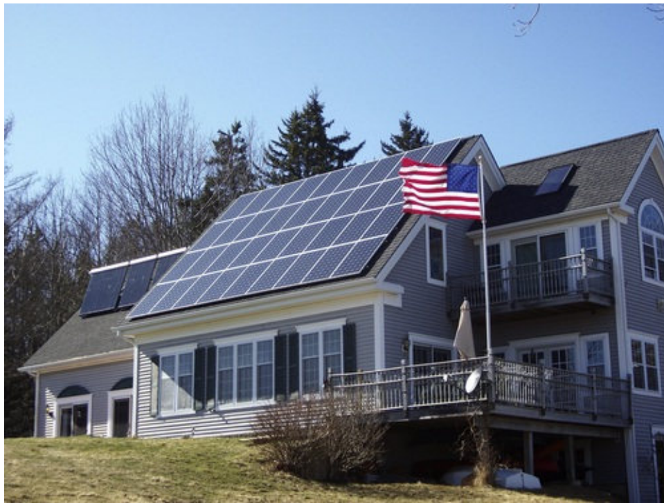
FIGURE 5.4 8.64 kW array composed of 36 Canadian Solar CSP6M
