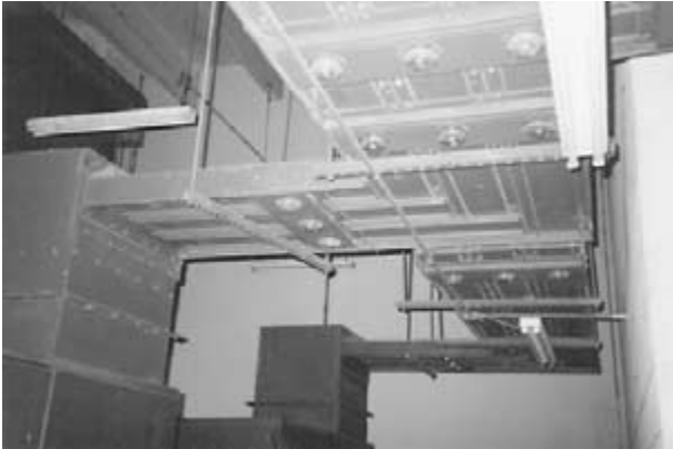
Bus duct is used to carry large values of current.
