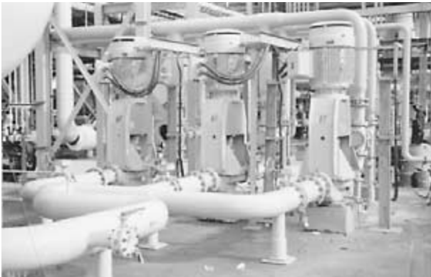
Induction motors driving pumps in industrial facility.
