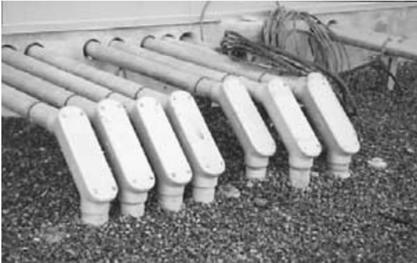
Condulet fittings are used to turn short-radius bends.
