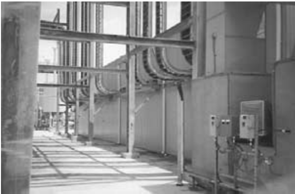
Cabling in a cable tray is a normal wiring method in industrial facilities.
