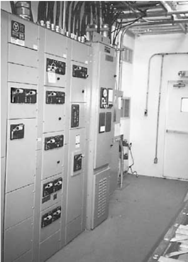
Motor control center.
