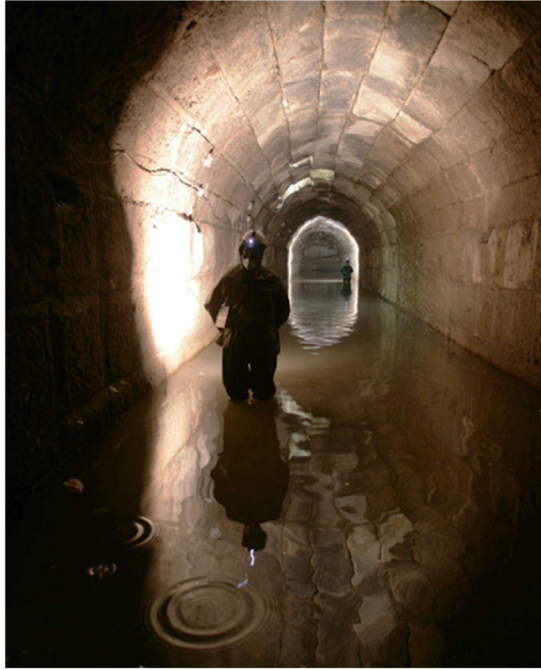
Figure 1.10 A worker inspecting a 6th century drainage tunnel still in use today in Rome (Alvarez, 2006).
