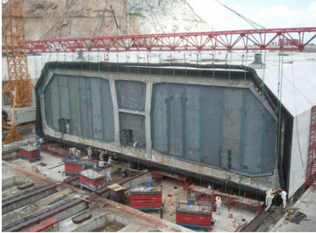
Figure 4.74 Installation of a continuous rubber gasket. Courtesy of Hong Kong Zhuhai Macao Bridge Authority.
