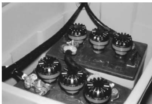
FIGURE 11.11 Catalytic recombiner caps used on deep-cycle LA batteries for a PV system. Note the rubber container to contain any possible acid spills and appropriate battery cables.
