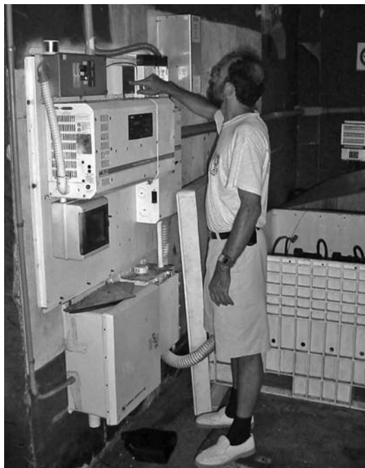
FIGURE 8.25 Isla Contoy solar and wind energy power center, inverter, controls, and batteries.
