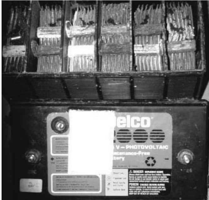
FIGURE 11.10 Excessive plate sulfation and buckling as a result of consistent undercharging of a battery in Ceara, Brazil, for a small residential PV home system.
