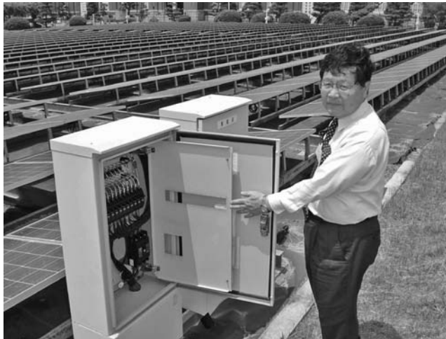
FIGURE 8.5 Project designer Mr. Ohashi and Osaka Waterworks Kunijima Treatment Plant with a 150 kW p PV plant (Kyocera), one of over a dozen such PV water plants in Japan.
