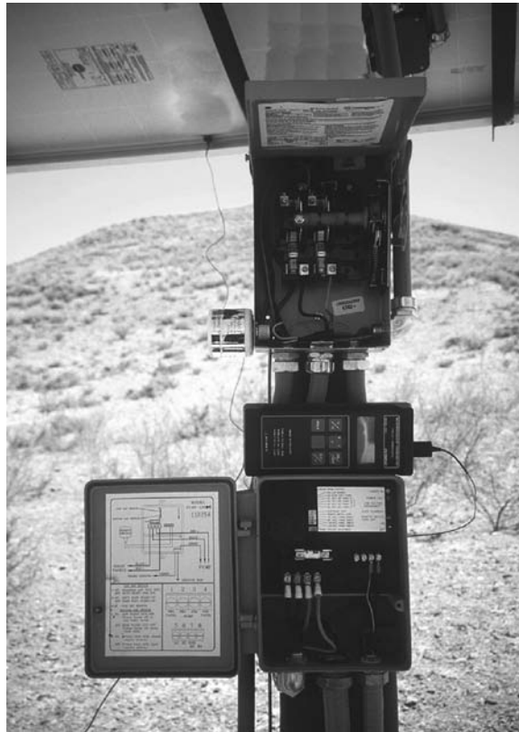
FIGURE 8.39 Typical pump controller with overcurrent protection for PV water-pumping system in Chihuahua, Mexico.
