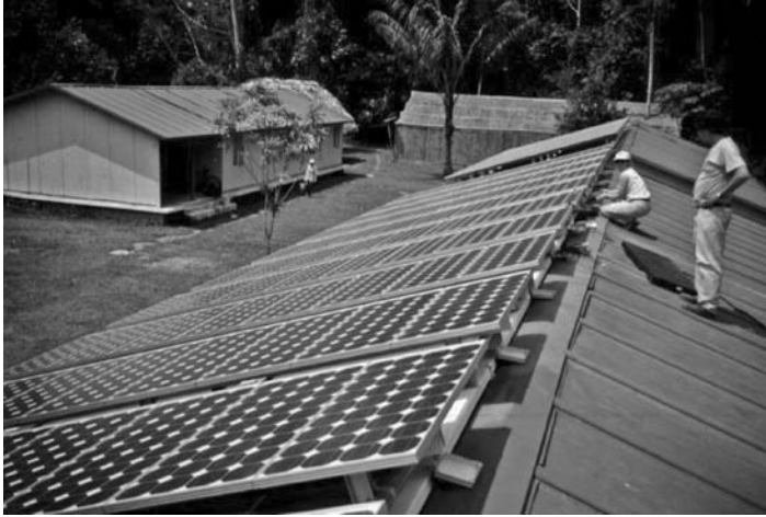
FIGURE 7.3 Mexico's first NEC -compliant PV system installed at Montes Azules Biosphere Reserve in Chiapas (1998) by WWF/USAID, Conдумex, Sandia, and NMSU.
