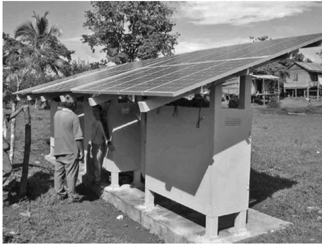
FIGURE 8.19 One of the three PV battery charging stations (NW system) at Francia Sirpi, Nicaragua.
