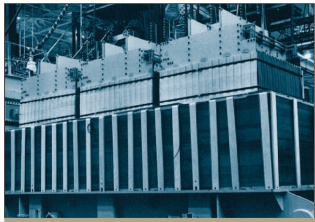
FIGURE 18-28 Core of a 600-MVA three-phase transformer. Courtesy of Houston Lighting and Power.
