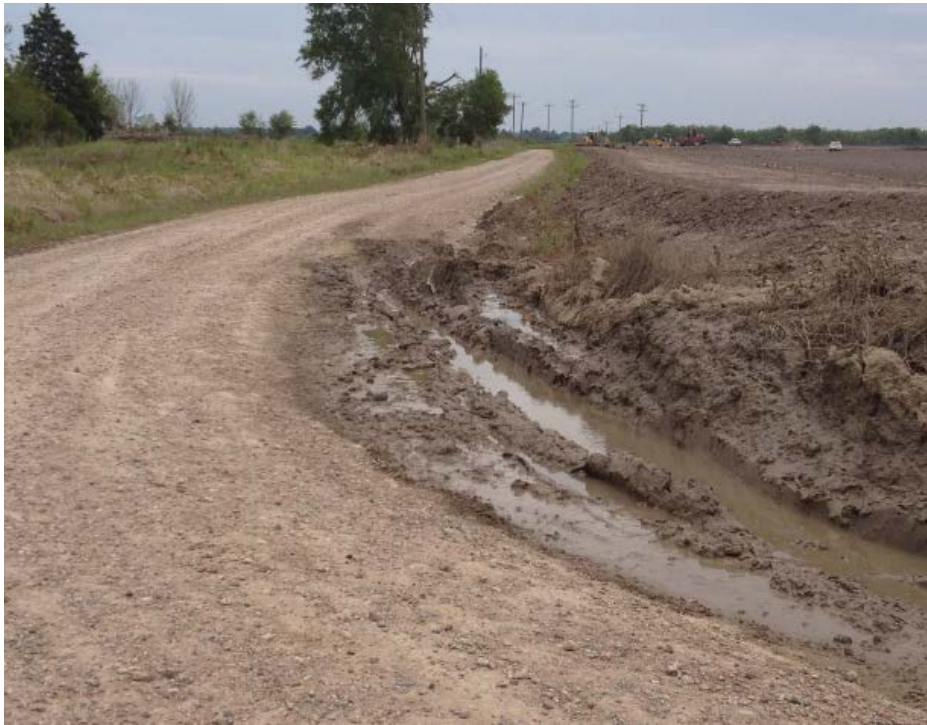
Lack of ditch drainage affects the performance of this road.
