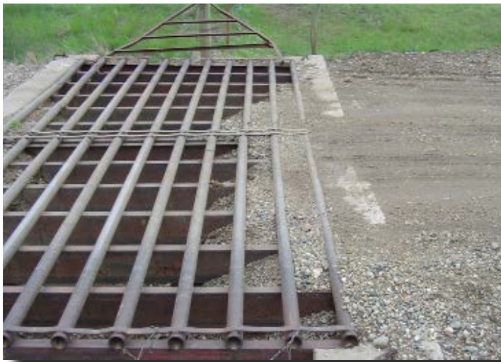
Care must be taken not to spill gravel into the cattle guard. Poor quality gravel with too much loose aggregate aggravates the problem of material spilling into the cavity spill gravel into the cattle guard.
