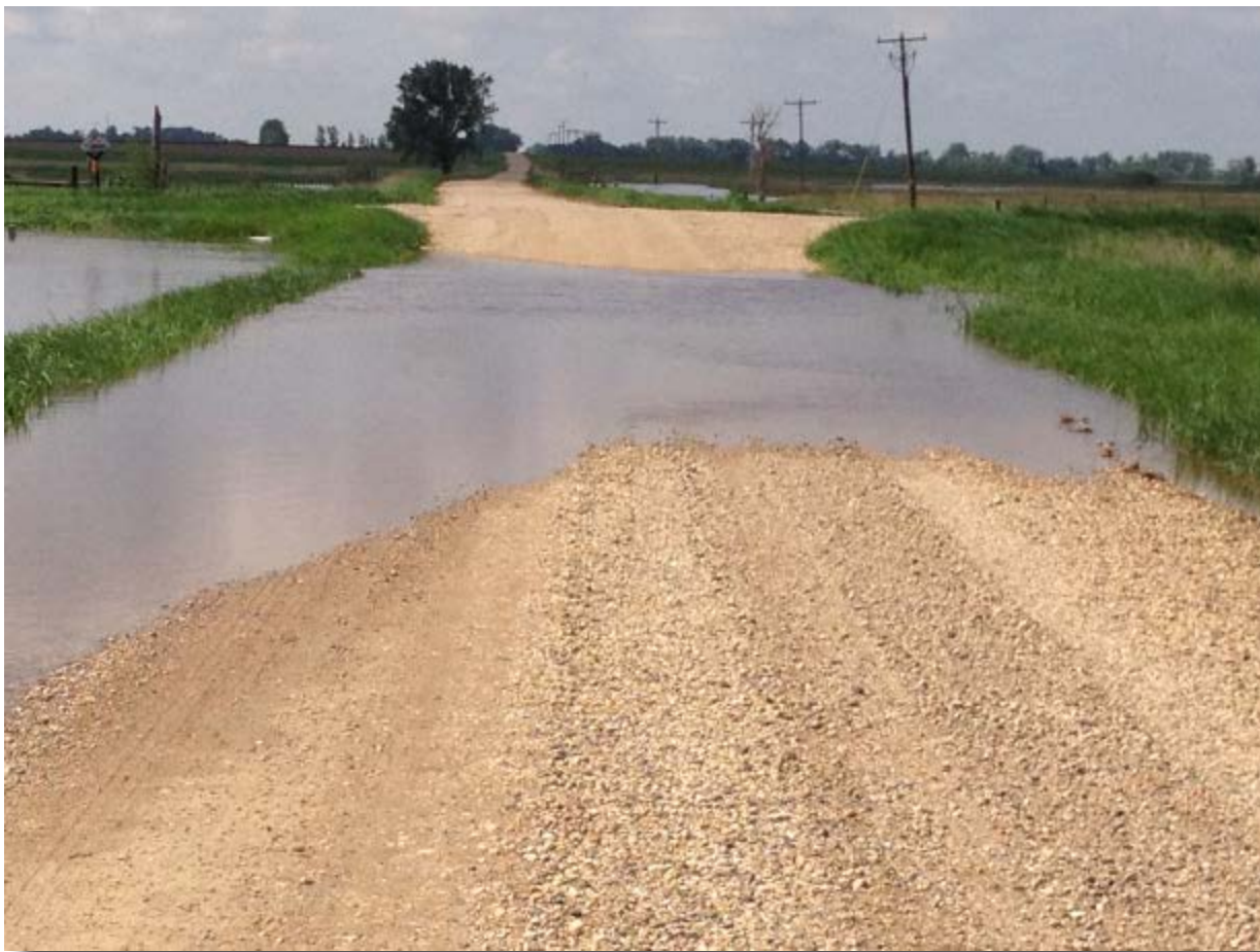
Plugged or collapsed culverts cause serious damage when water flows over roads.
