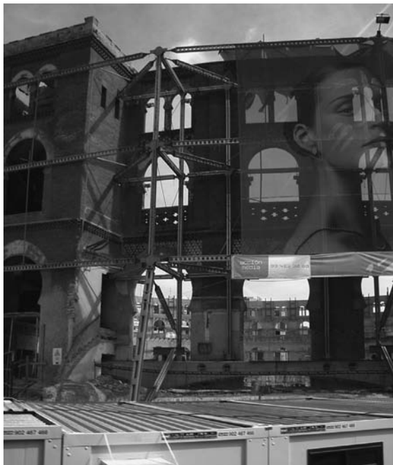
Photograph 13.9 Proprietary adjustable façade retention system
