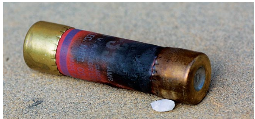
Burned areas normally signify a loose connection on the fuse holder or within the panel.
