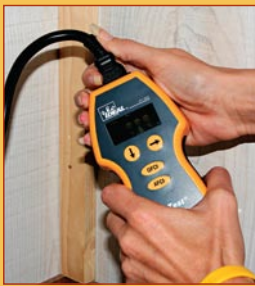
203 | Troubleshooting an AFCI Circuit
