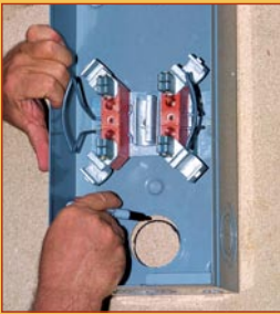
66 | Locating the Meter Base
