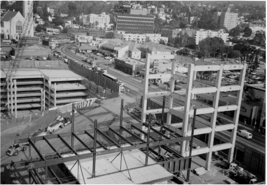
Photo 3.5 Precast DDC frame tower, Hollywood Highland Project, Hollywood CA. (Courtesy of Englekirk Partners, Inc.)
