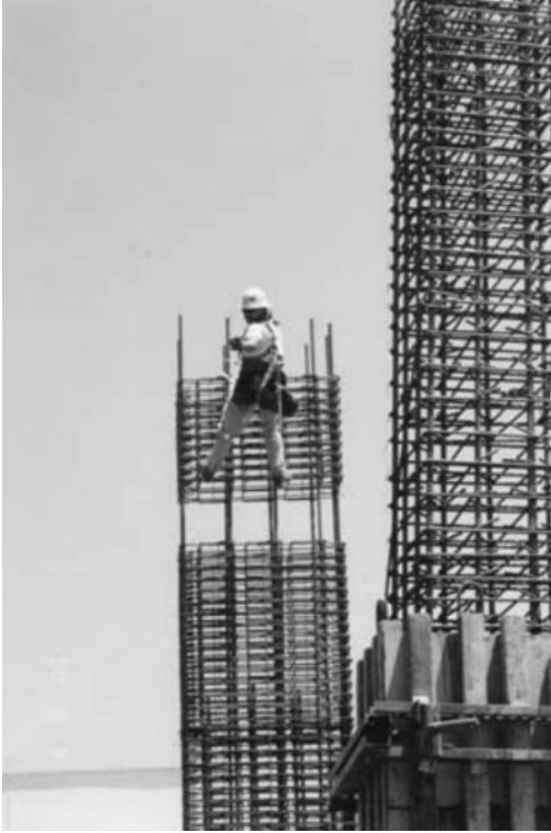
Photo 3.3 Placing a two-story column cage, The Remington, Westwood, CA. (Courtesy of Morley Construction Co.)
