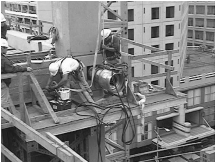
Photo 2.5 Preparing to stress a hybrid frame beam, Paramount Apartments, San Francisco, CA. (Courtesy of Charles Pankow Builders.)
