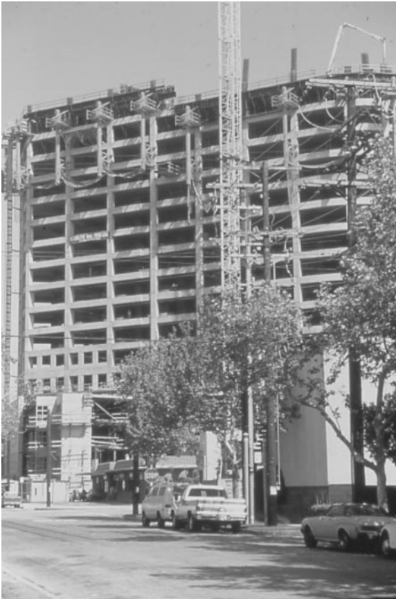
Photo 3.2 Cast-in-place concrete ductile frame construction, jump form framing. (Courtesy of Englekirk Partners, Inc.)
