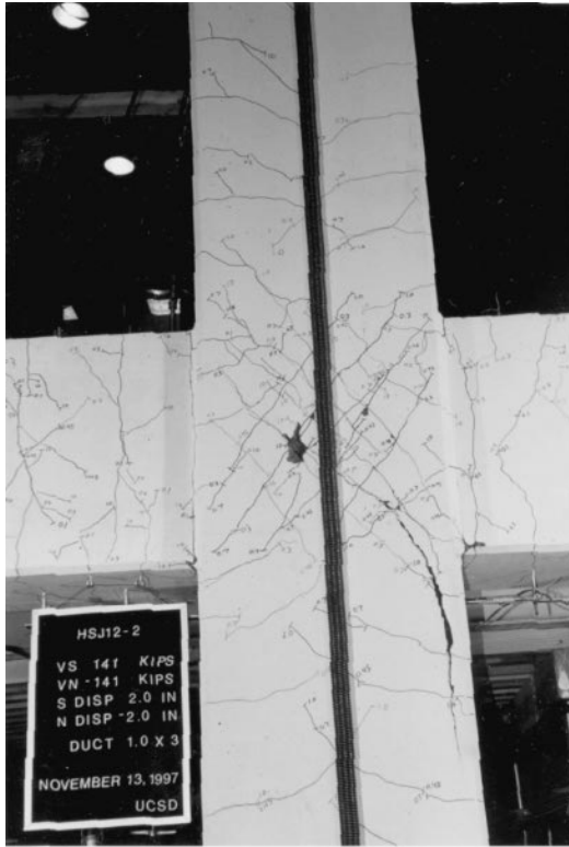
Figure 2.3.2 Joint shear cracks are widening and extending. The cover has begun to spall.
