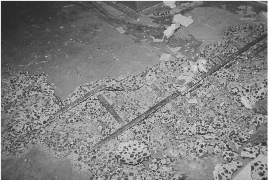
Photo 1.4 Flat slab with shear head shear failure, Northridge earthquake, 1994. (Courtesy of Englekirk Partners, Inc.)
