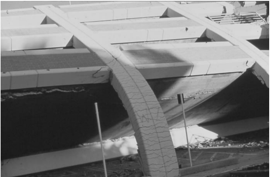
Photo 1.1 Ductile concrete, Northridge earthquake, 1994. (Courtesy of Englekirk Partners, Inc.)
