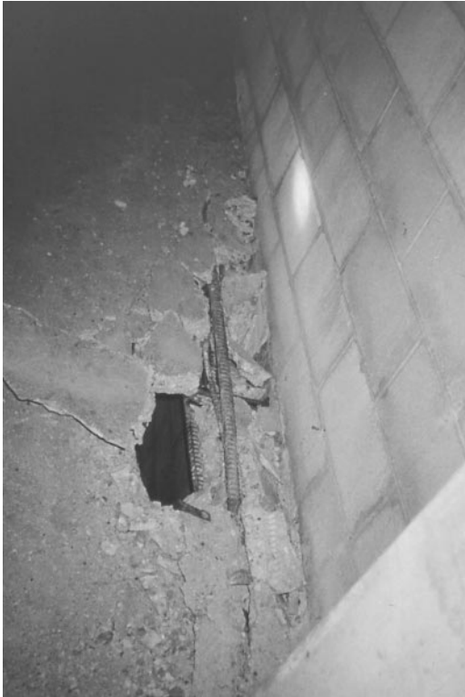
Figure 3.3.5 Buckling of chord bars in a diaphragm.
