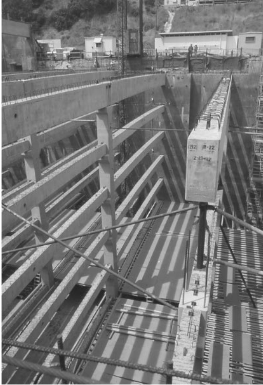
Photo 3.4 Nine-story precast concrete column, Getty Center Parking Structure, Brentwood, CA. (Courtesy of Englekirk Partners, Inc.)
