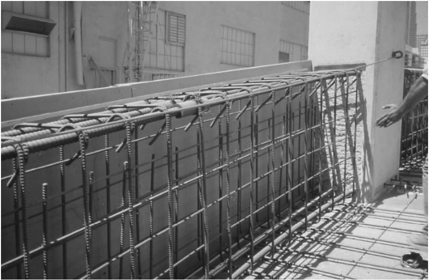
Photo 2.3 Composite frame beam, DDC connection to precast column, Staples Parking Structure, Los Angeles, CA. (Courtesy of Englekirk Partners, Inc.)
