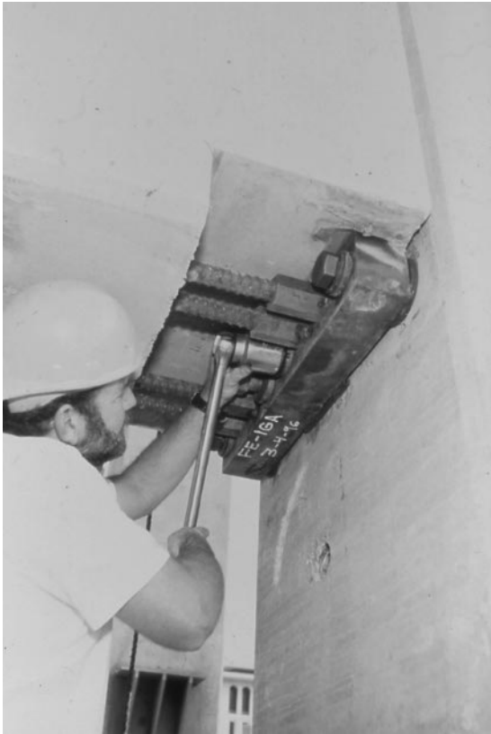
Photo 2.6 Assembling a DDC frame beam, Wiltern Parking Structure, Los Angeles, CA. (Courtesy of Englekirk Partners, Inc.)
