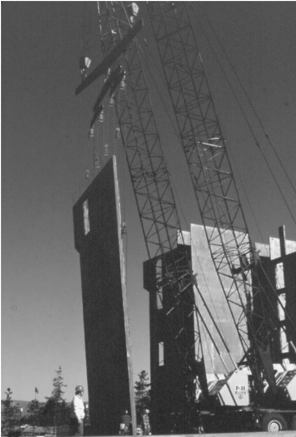
Photo 2.9 Six 6-story precast concrete wall panels, Hilton Hotel, Oxnard, CA, 1968. (Courtesy of Englekirk Partners, Inc.)
