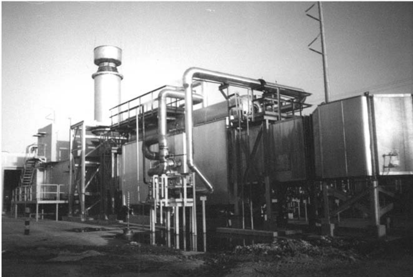
FIGURE 1.14b Photograph of a furnace-fired ABCO HRSG in a cogeneration plant.
