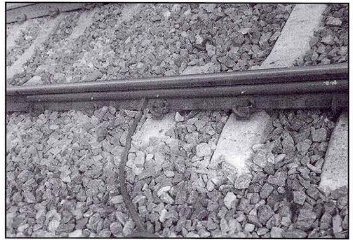
Fig. 13.4 Flat wheel detector (WILD) [Load circuits with strain gauge patterns mounted in the web of the rail and covered by a plastic cover]
