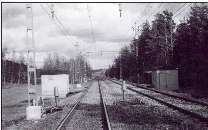
Fig. 13.3 Detector site in Sweden with profile supervision detector, hot wheel detector and hot box detector
