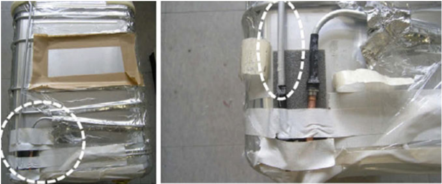
(a) Pitted evaporator tube in field
