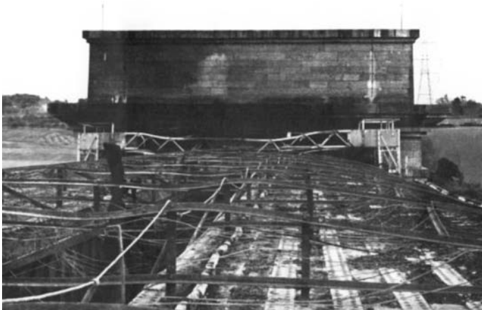
Fig. 13.13 The burnt-down roof of the Britannia Bridge. ( www.2d53.co.uk/britanniabridge/menu.htm )
