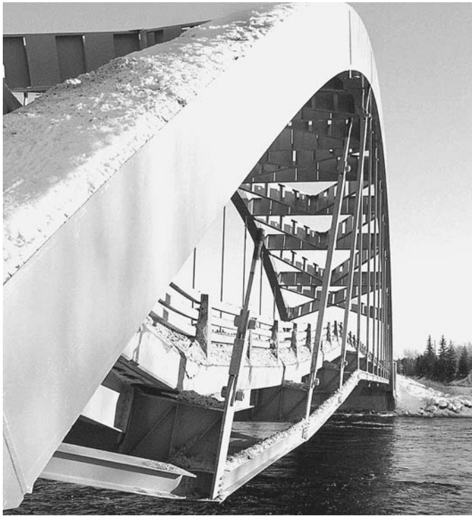
Fig. 20.15 The (partial) collapse of the Sgt. Aubrey Cosens VC Memorial Bridge. ( http://speaker.northernontario.ca/content/Feature%20Story/C%20Front%2011:01:06.pdf )
