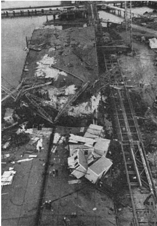
Fig. 15.18 The collapsed girder span on the ground. (Report of Royal Commission into the Failure of West Gate Bridge. Copyright State Government of Victoria, Australia)
