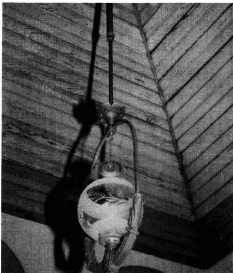
Fig. 8-16. This old light fixture has been rewired.
