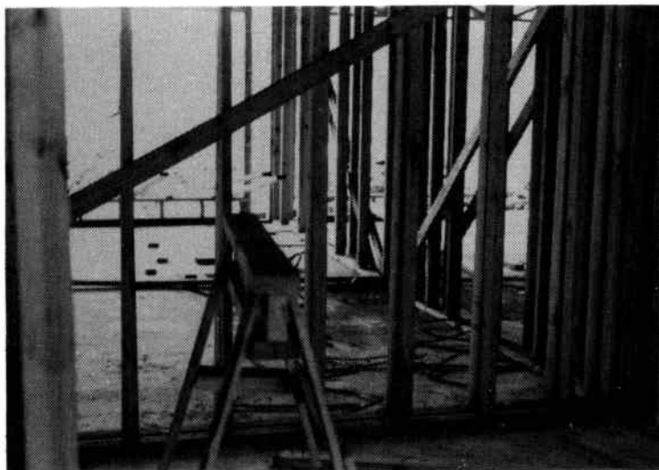
Fig. 6-2. Inside of a home under construction. The walls have been framed on a cement slab and the roof is in place.
