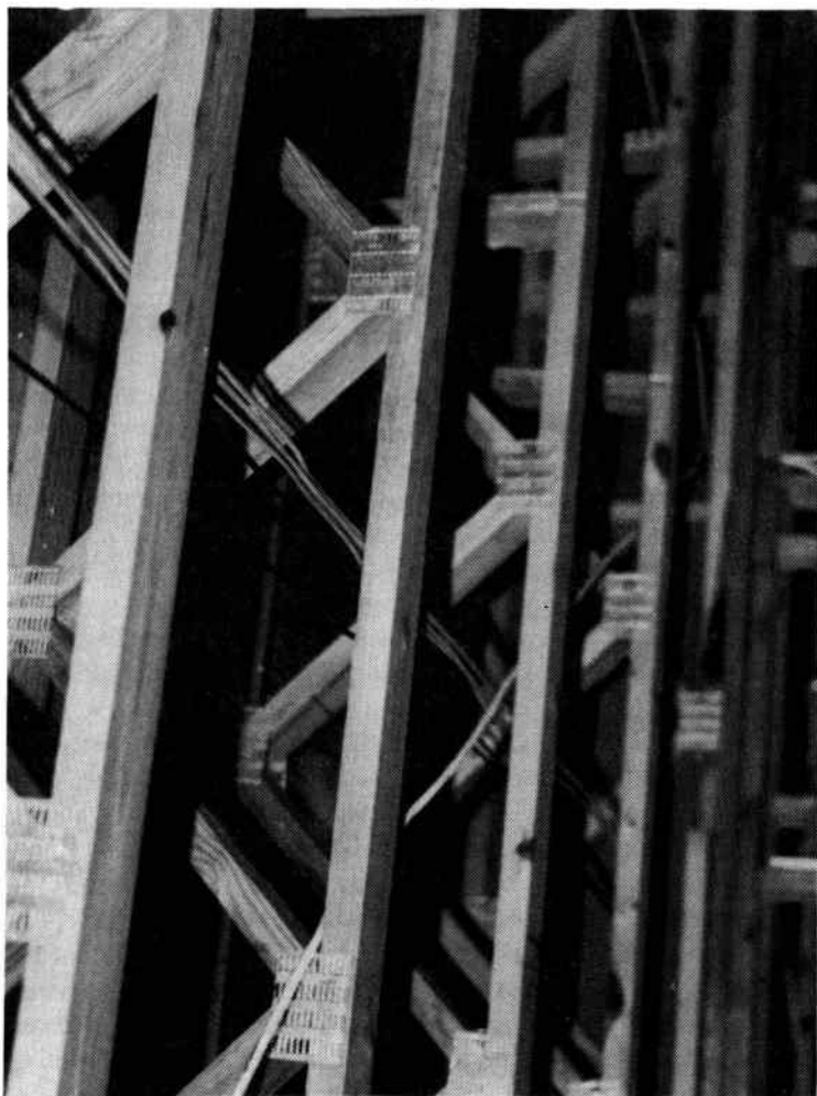
Fig. 6-18. Cables can be run over the ceiling beams in the crawl space or in the attic.
