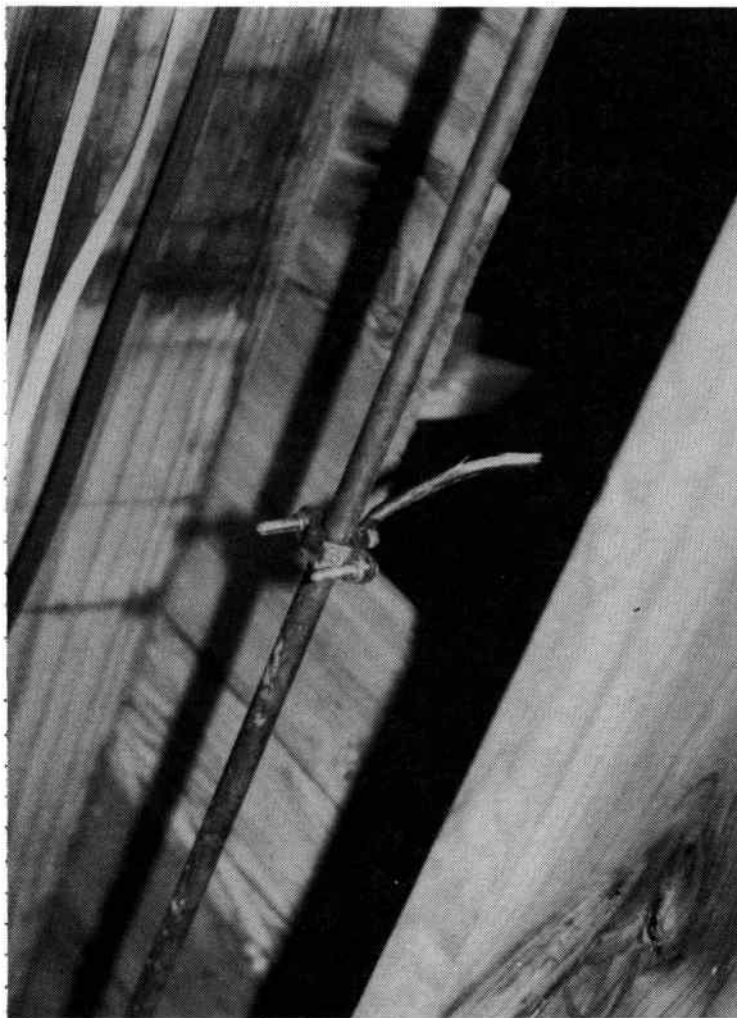
Fig. 3-8. Connection to a copper water line for grounding.
