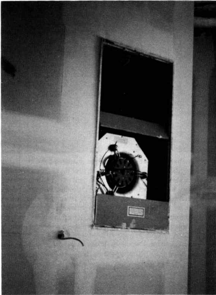
Fig. 5-18. A small internal air conditioning unit.
