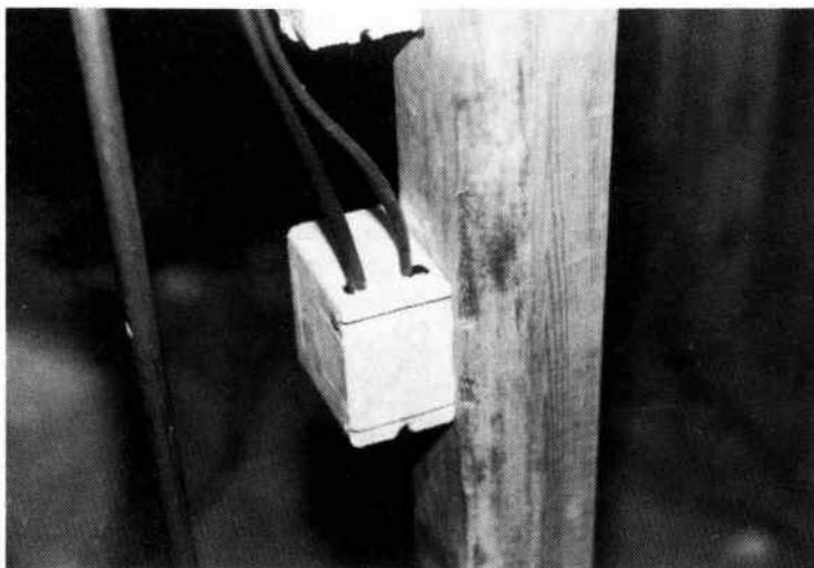
Fig. 6-44. Romex going into a plastic box uses no fittings.
