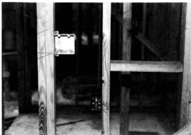
Fig. 6-14. Rough-in of a switch box and receptacle box on adjacent studs. The horizontal "V" shows the height at which the box is to be set.
