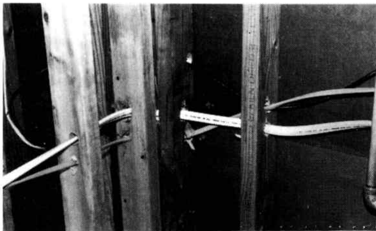
Fig. 6-23. The routing of a large cable on a run along a kitchen wall as it goes to the utility room.
