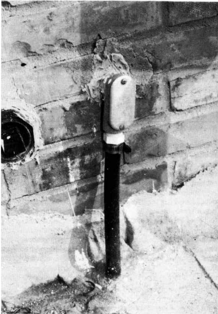
Fig. 2-7. Fittings on an underground electrical wiring installation from a house to the garage.
