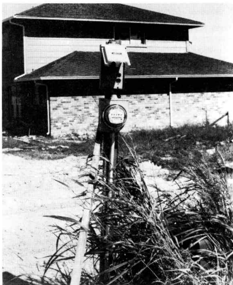
Fig. 8-18. Temporary service connection to an underground conduit provides power to run electrical tools.
