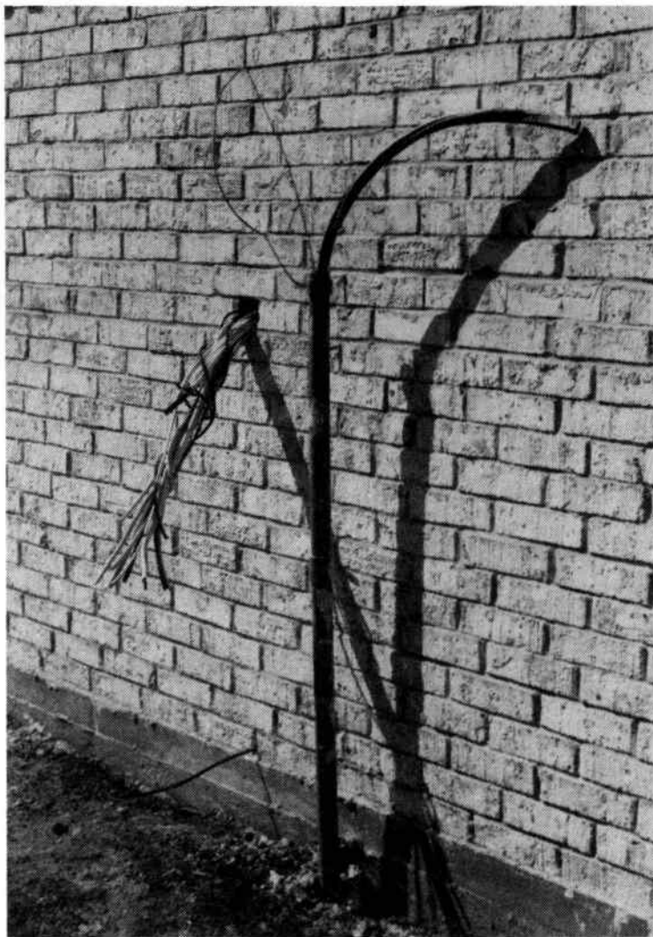
Fig. 6-60. Circuit breaker panel wires and cables are shown along with the location of the electric meter socket. The underground riser of the service feed is also shown to the right.
