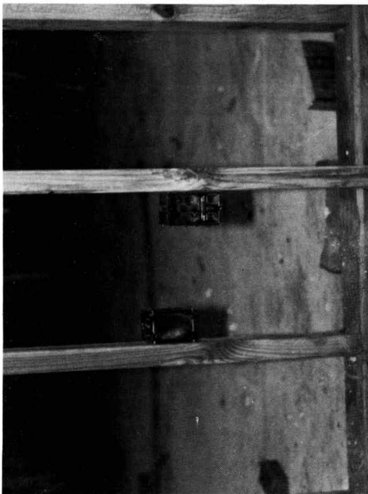
Fig. 6-12. Two back-to-back boxes on adjacent studs. These may not be wired on the same branch circuit.
