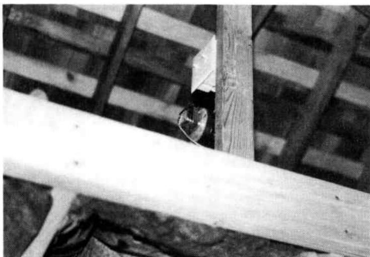
Fig. 6-35. Bell transformer and attic switches.
