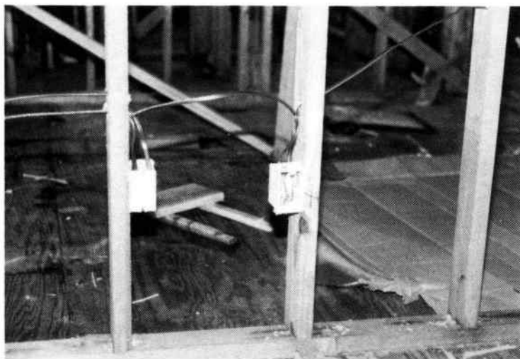
Fig. 6-45. The wiring of back-to-back boxes on adjacent studs. Several branch circuits are involved.
