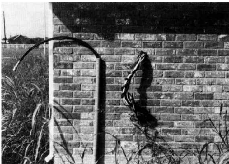
Fig. 6-70. Meter and circuit breaker panel location for a new home. The service riser is to the left.
