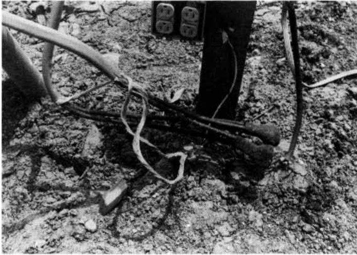
Fig. 3-18. Notice the method of connection to electric lines. A clamp is used on neutral bare wires.
