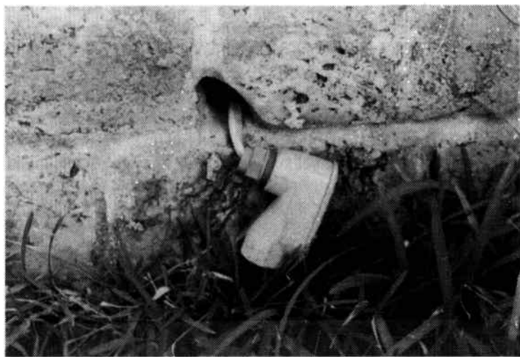
Fig. 7-15. A dangerous outside connection.
