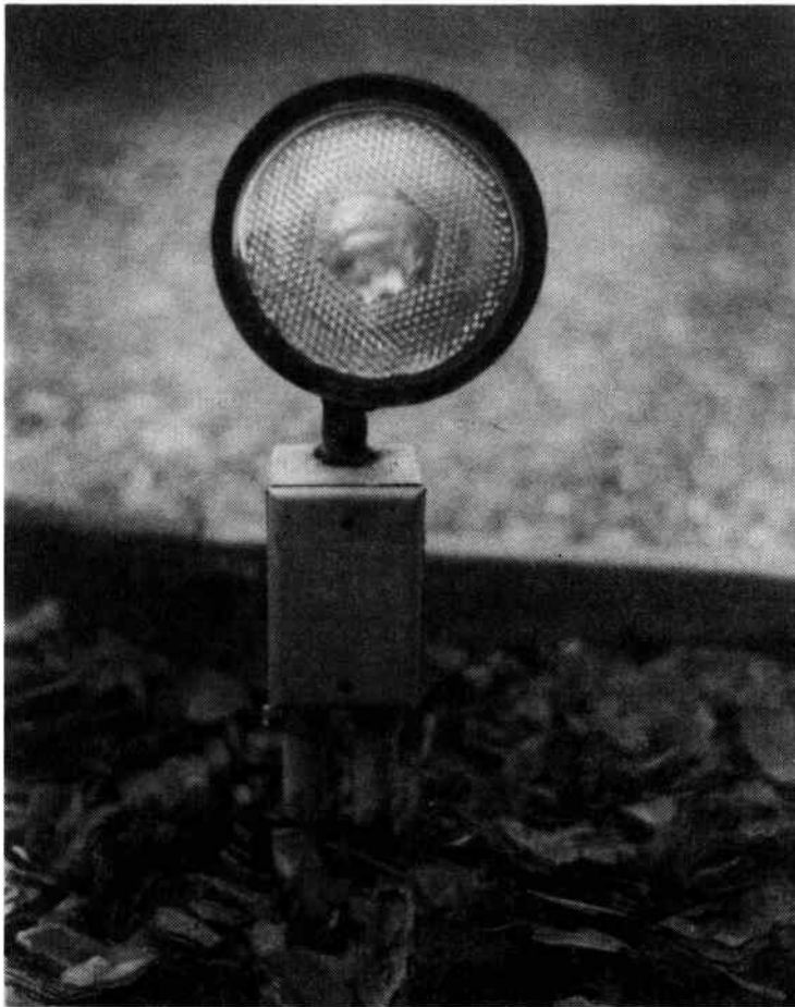
Fig. 7-11. The conduit for this fixture is metallic.
