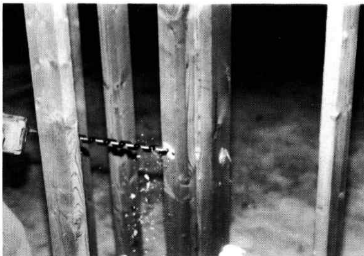
Fig. 6-16. Going around a corner in the framing means lots of holes. Holes must be centered at least 1½ inches from the edge of the studs so nails will not pierce the cable.
