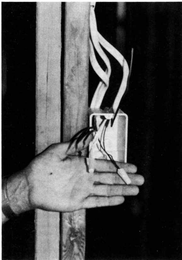
Fig. 4-4. Electrical nut insulators and connectors cover the ends of the twisted wires.
